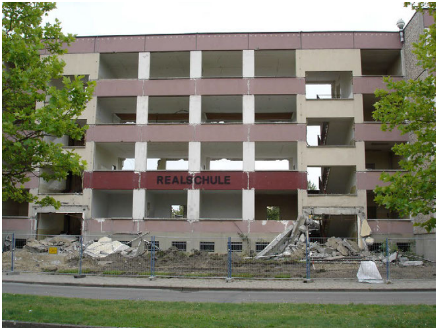
Picture 4: Symbols of the population decrease in Eastern Germany, demolition of a school building in Wittenberge (Source: Benno Brandstetter).
