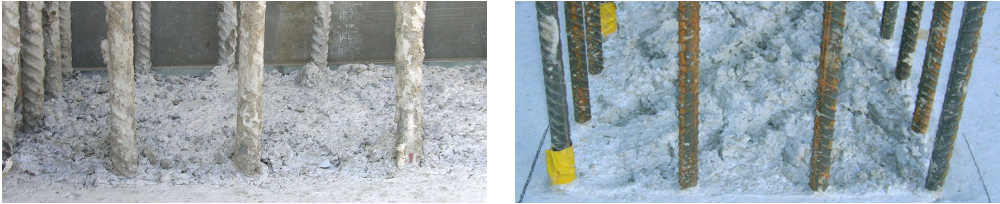
Figure 2.5: Pictures of the construction joints of VK4 (left) and VK5 (right). Construction joints of VK6 and VK7 were treated in the same manner.
