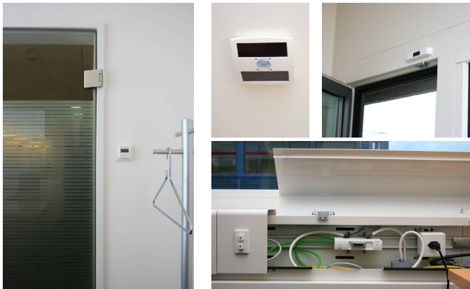
Fig. 2 Additional equipment installed in offices: wireless room temperature sensor (left, next to the office door), wireless presence and illuminance sensor (top middle, at ceiling), wireless window contacts (top right, above the window), electrical energy meter for measuring consumption for illuminance (bottom right, within the media channel).
