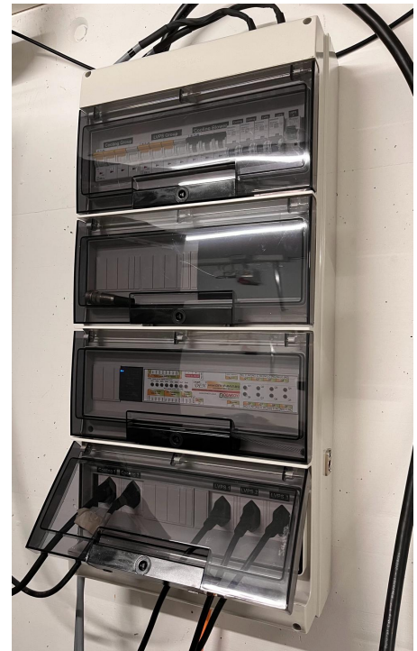
Figure 3.1: Image of the power control panel.
