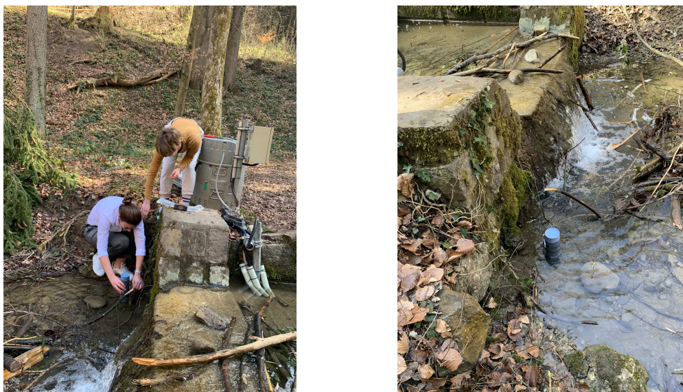
Figure A.4: LEFT: Students installing the simple turbidity sensor in the Holderbach. RIGHT: The installed sensor in the Holderbach.
