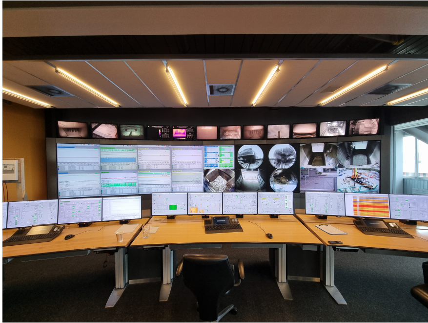
Figure 1.1. ERZ Hagenholz control room Zürich, Switzerland, 24.05.2024.
