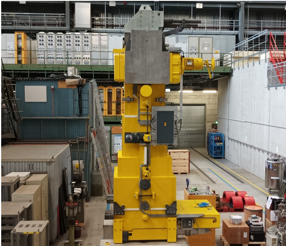
Figure 5.7: TgE remote-handling exchange flask in the HIPA facility experimental hall.
