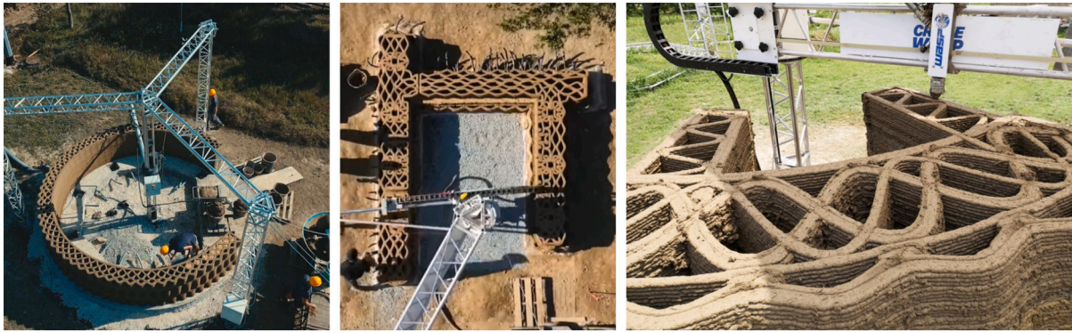
Fig. 7. Different large-scale projects for two-story houses have adopted significantly different geometry and shapes of printing paths. On the left, Gaia Project by Wasp [55], Tova project by IAAC [74] (middle) and the Tecla House (right) [34].
