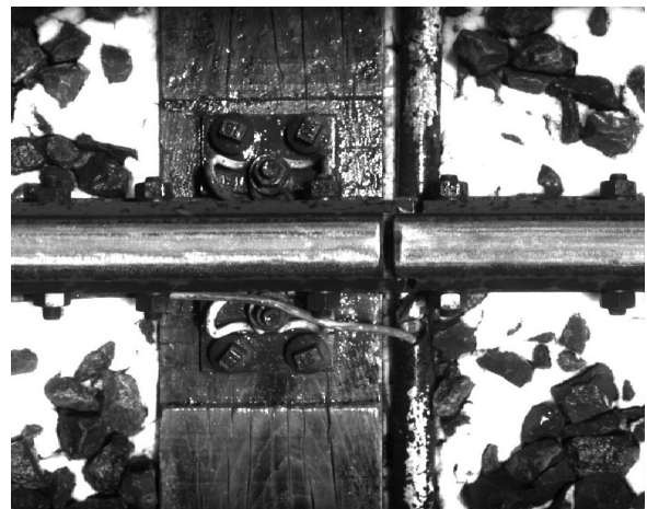
(b) Joint with broken joint plate
