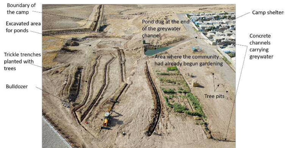
Fig. 09: The SuDS management train under construction in the Gawilan Refugee Camp, Kurdistan Region of Iraq. Charlesworth et al. 2019, p.3505.
