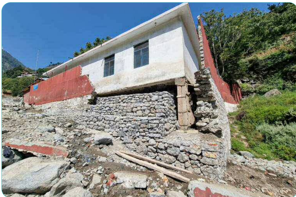
Fig. 07: Torwal school in the Swat Valley, Pakistan. Rehabilitation works with gabion walls. Christian Neuhaus, SDC 2022.
