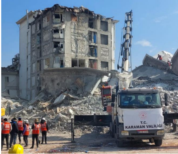
(a) Post-earthquake view from the west of the hospital ( Twitter ), showing minimal structural tie-in between the collapsed and still standing portions of the northwest wings of the hospital.
