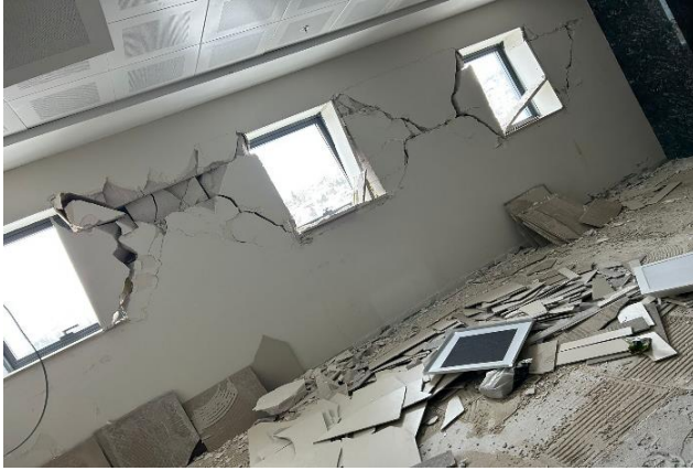
(a) Façade walls and falling of ceiling tiles.
