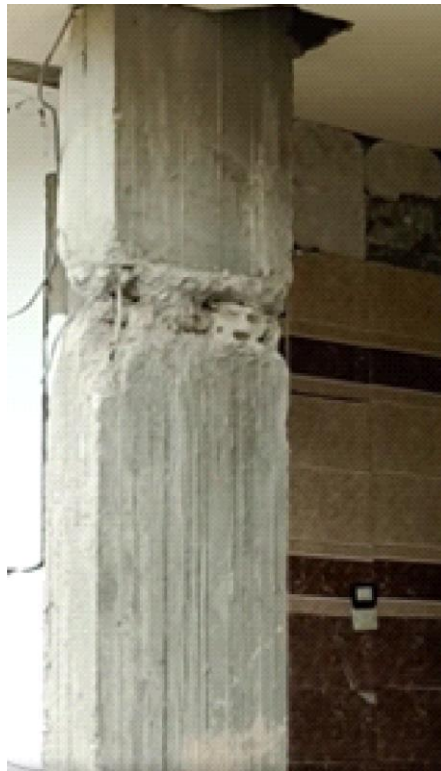
Figure 3.3. Damaged RC column with severe deficiency of reinforcement (Source: Personal image by Eng. M. Zakaria member of damage assessment commission).
