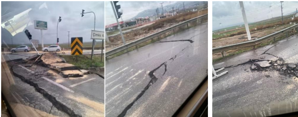
Figure 5.2. Surface failure of roadway (Source: Channel News Asia ).
