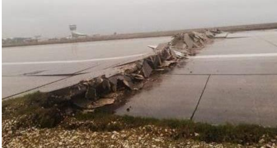
Figure 5.7. Hatay Airport in southeastern Türkiye has suspended operations due to runway damage caused by the earthquake sequence (Source: Twitter ).
