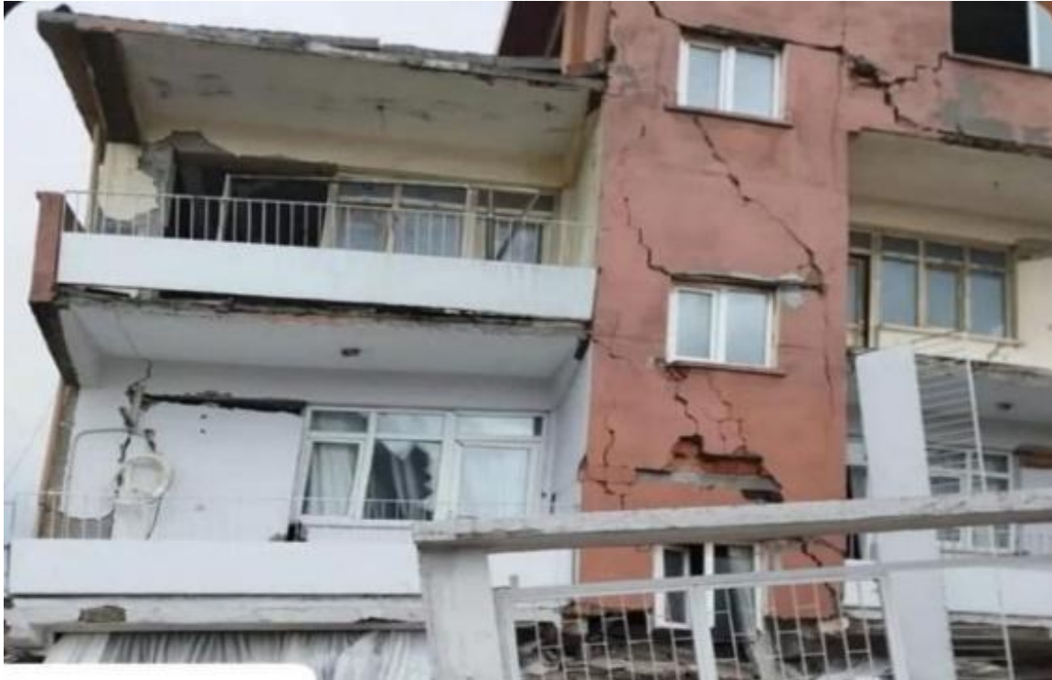
Figure 4.73. Examples of nonstructural components (bricks and parapets), which can be a falling hazard, in a residential building in Hatay, Türkiye. It was also announced that residents were stuck in the stairwell (Source: Ozgur via Twitter 2023).
