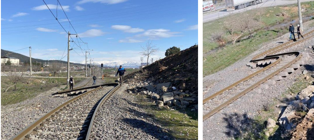
Figure 5.9. Deformed railway between Kahramanmaraş, Türkoğlu, and Gaziantep, İslahiye (Sources: Reddit (left) and Facebook (right)).
