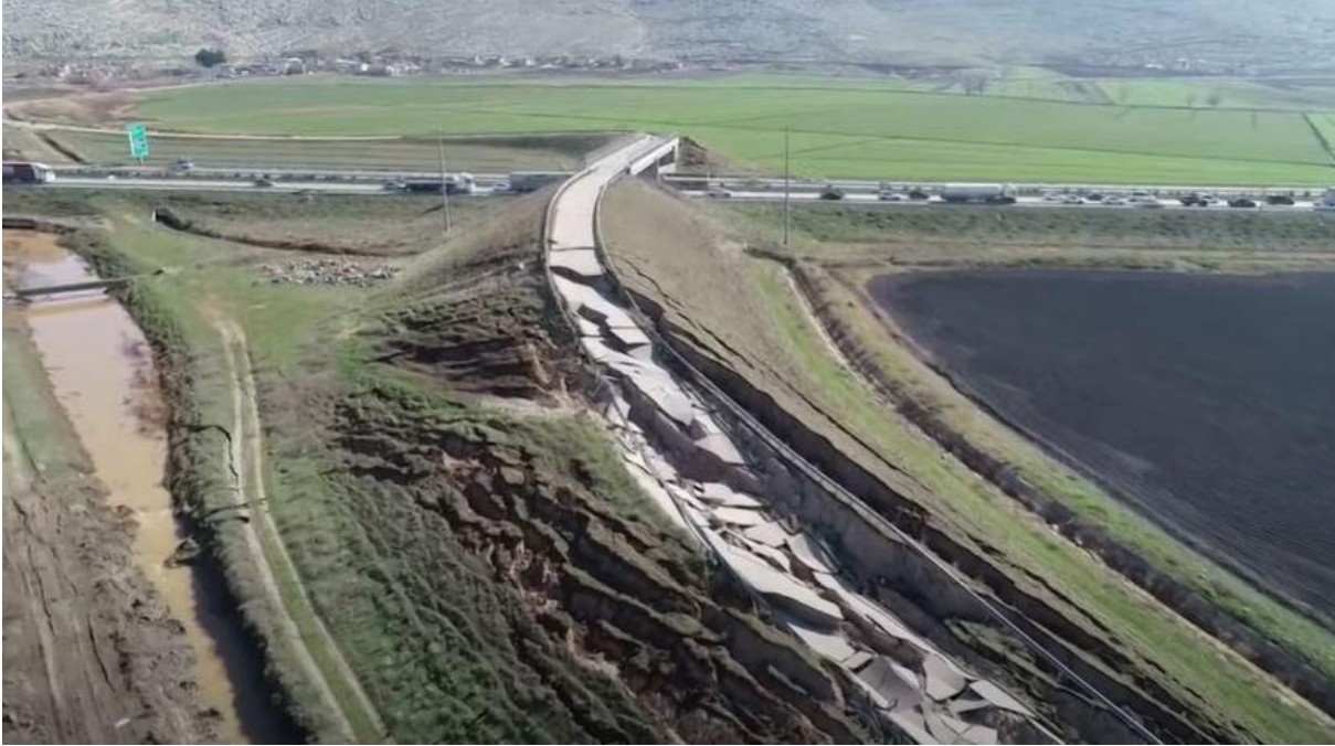
Figure 6.11. Failure of the embankment road in the village of Koseli, which passes over the Adiyaman-Sanlıurfa-Gaziantep Highway in the Adiyaman province (Source: Reuters via Washington Post ).
