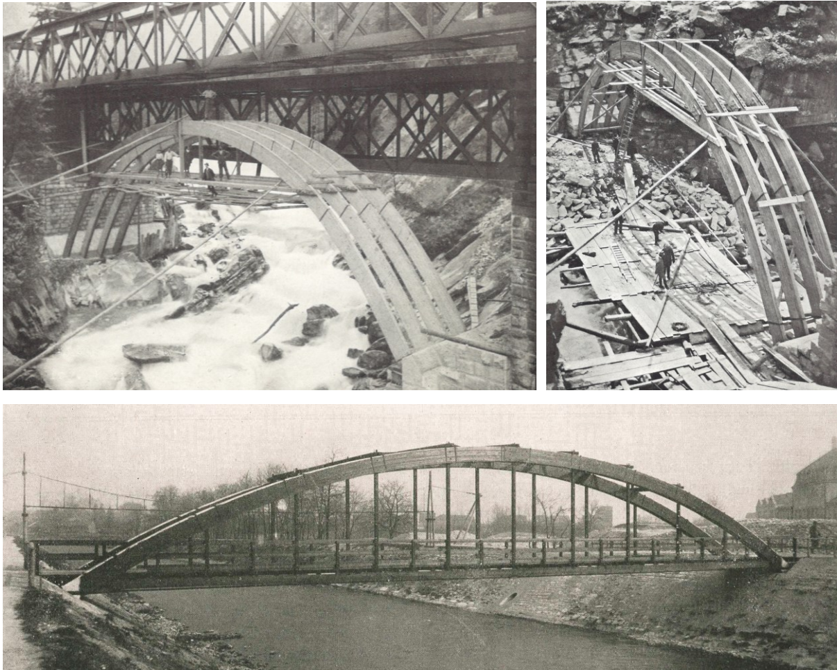
Fig. 6 Glulam formwork for a masonry bridge of Gotthard Railway, near Rodi-Fiesso, Ticino.
