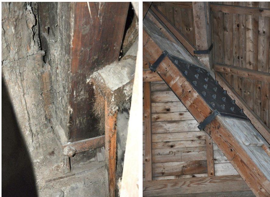
Figs 7-8 Details of the footing of a girder and a site joint. Visit in 2018.
