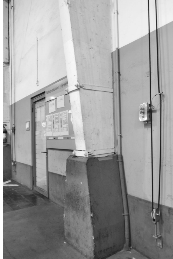
Fig 16 Locomotive depot, Bern. State of the base of one girder after the removal of the decayed section and its replacement by a concrete pedestal.
