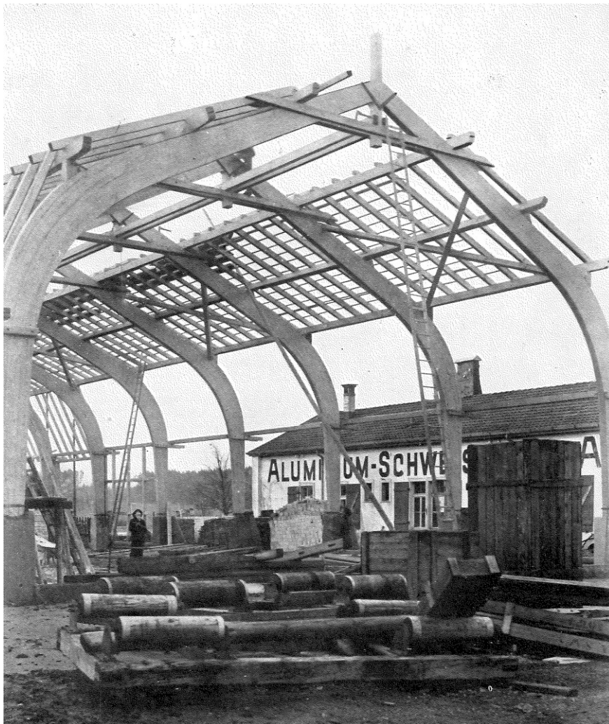
Fig. 58 Glulam structure of the workshop of the Aluminium Schweisswerk AG in Schlieren
