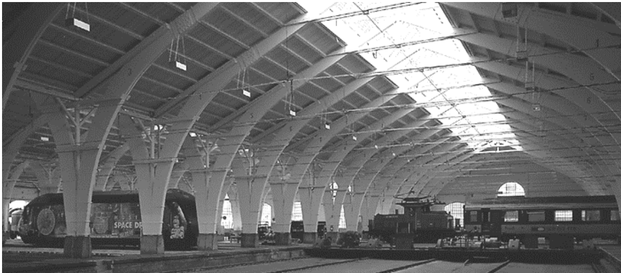
Fig. 11. Glulam structure of the locomotive depot in Bern, 1998. Due to the degraded condition of the structure, the glulam girders are now supported by wooden posts.
