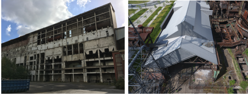
Figure 5.13: Buildings of the Gustav Knepper powerplant (left) and the Phoenix-West foundry (right).
