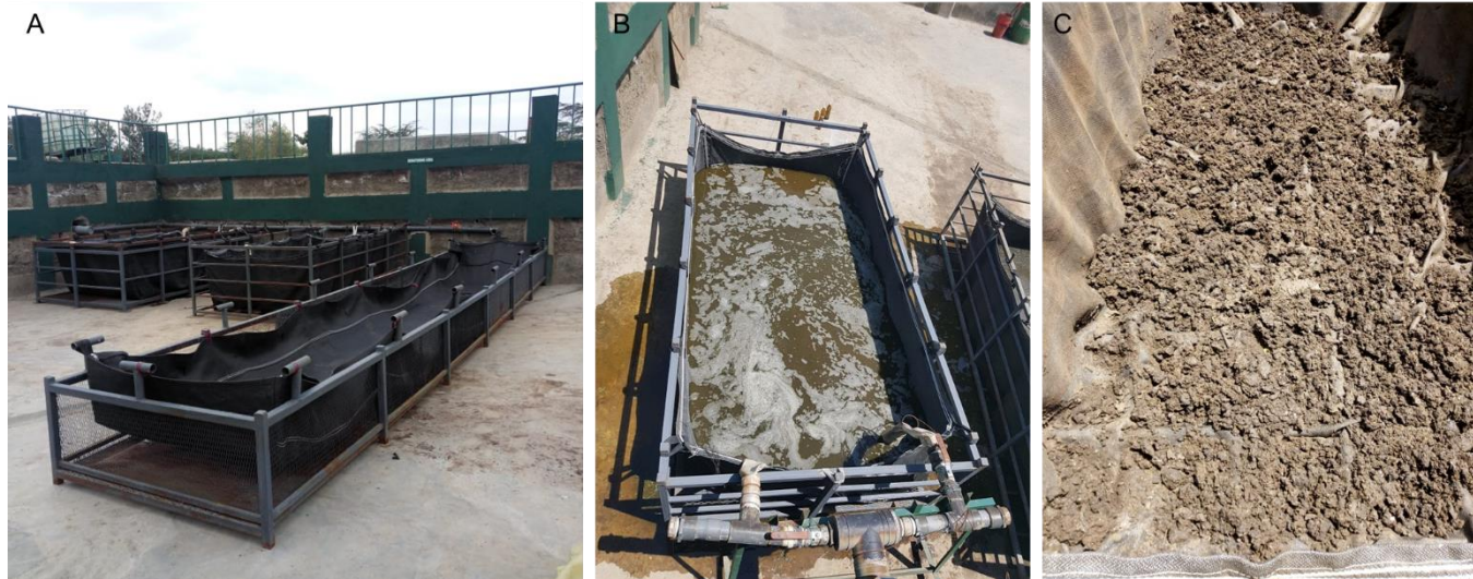
Figure 3.10. A) a geotextile skip setup at the pilot facility; B) a geotextile skip being loaded with conditioned faecal sludge; C) dewatered sludge ready to be unloaded from a geotextile skip (photos: Sanivation).
