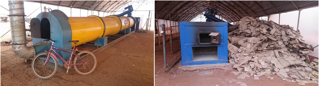
Figure 3.15. Left: a rotary convection dryer operated by Pivot, in Kigali, Rwanda and right: waste cardboard is burned in a boiler and the hot gases produced are used as the heat source for drying. The sludge is pre-dried by a solar dryer before entering the convective dryer pictured here (photos: UKZN PRG).
