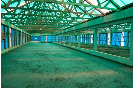
Figure 3.2. Settling-thickening tanks at Lubigi FSTP in Kampala, Uganda (photo: Sandec).
