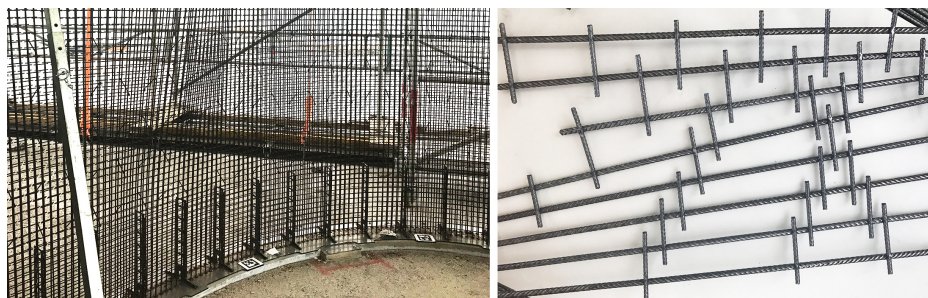
FIGURE 4.11: Insertion Experiments. Left: the regular-spaced straight bars in the Mesh Mould project; Right: the fabricated experiments to obtain data for the computational system.
