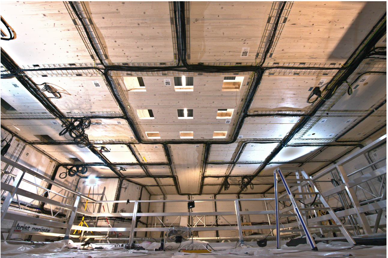
(c) Photo of the AMS while still under construction, taken from top of the MSR. At this point in time less than half of the coils were installed.
