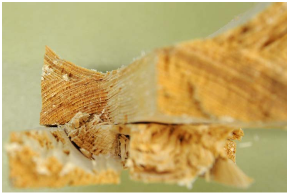
(e) failed section ( l \approx 4.8 m)
