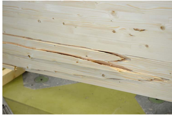
(b) back side ( l \approx 5.0 - 6.1 m), upper crack from 2nd failure cycle
