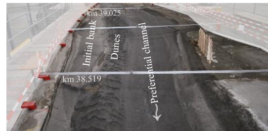
Figure 2: Verney widening at the end of 100-year flood test run (upstream view).
