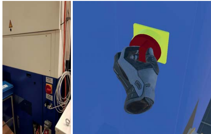
Figure 5 Real main switch for the power supply and the virtual twin (see online version for colours)
