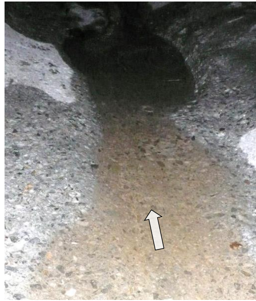
Figure 12: Erosion channel on the normal tunnel lining, picture taken 2012
