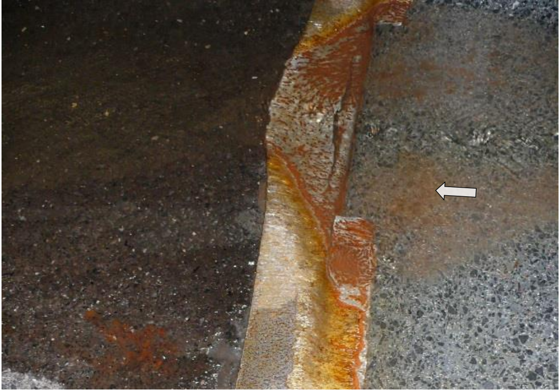
Figure 14: Damage on the steel beam separating the HPC field (right) from the SFC field (left), basaltic aggregates (dark grains) are visible, picture taken 2012
