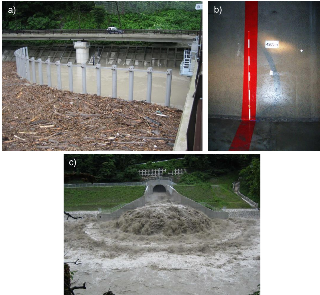
Figure 9: Situation of each facility in sediment bypass, a) log boom during flood, b) inner wall of tunnel after flood, c) energy dissipator during flood
