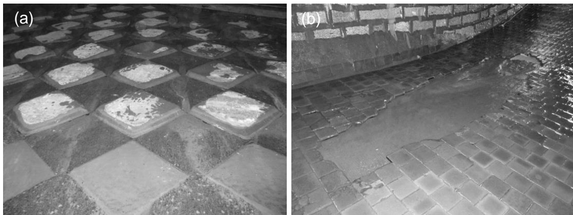
Figure 9: Abrasive wear in flow direction and local damage. (a) Diagonally checkered cast basalt tiles with mortar panels in between, (b) field of subsequently scoured and washed out cast basalt tiles
