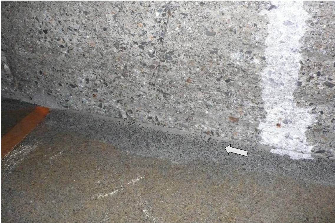
Figure 16: Minor damage due to abrasion in the PC test field and at the lower part of the wall (normal concrete), picture taken 2012
