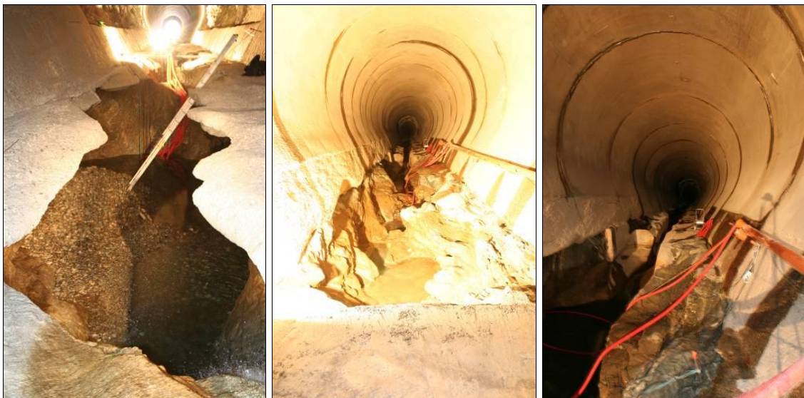
Figure 2: Eroded invert concrete and underlying Gneiss rock (2011)
