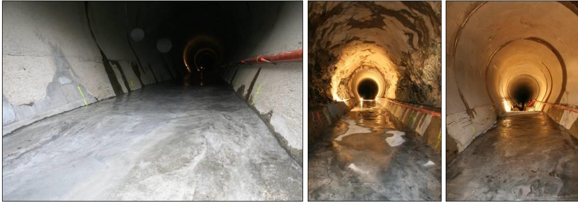
Figure 6: New concrete invert in the most downstream 350 m of the Palagnedra SBT (2013)
