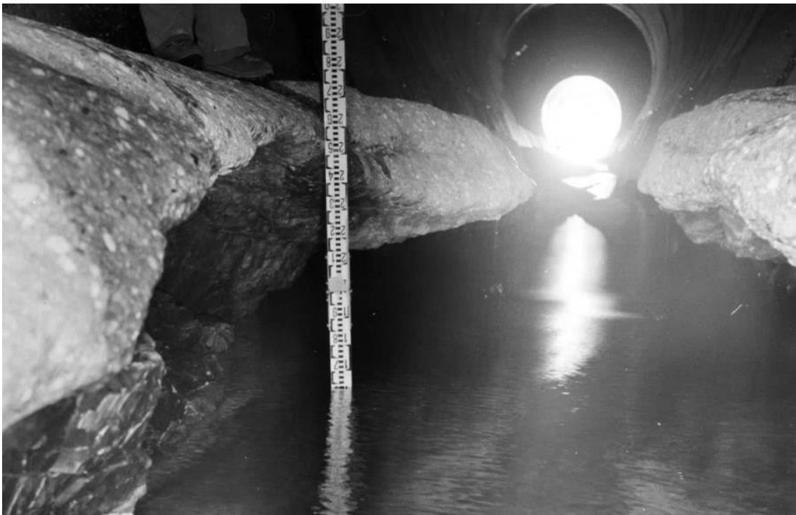
Figure 1: Invert damages at the Palagnedra SBT (Canton Ticino, Switzerland) after an exceptional flood event in 1978 (IM Maggia Engineering AG)
