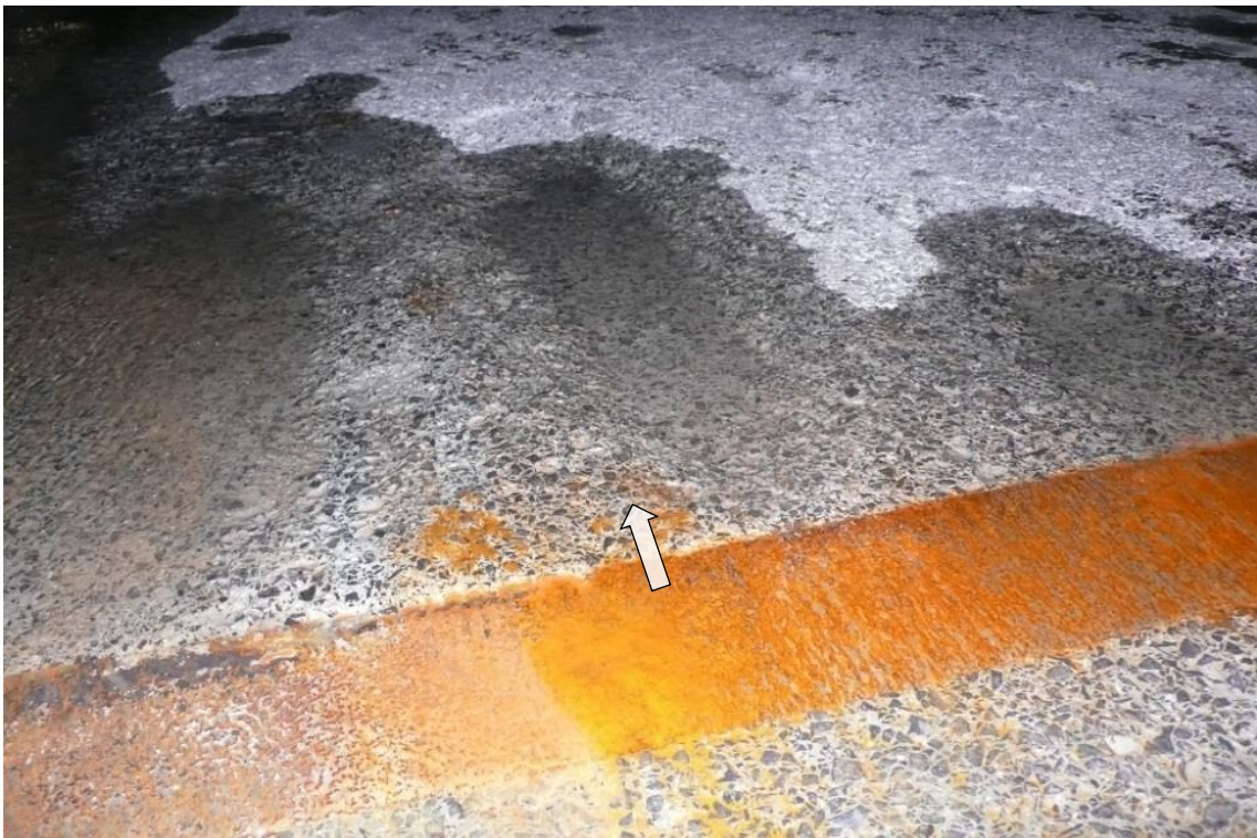
Figure 13: damage (uneven surface) in the HPC test field, picture taken 2012
