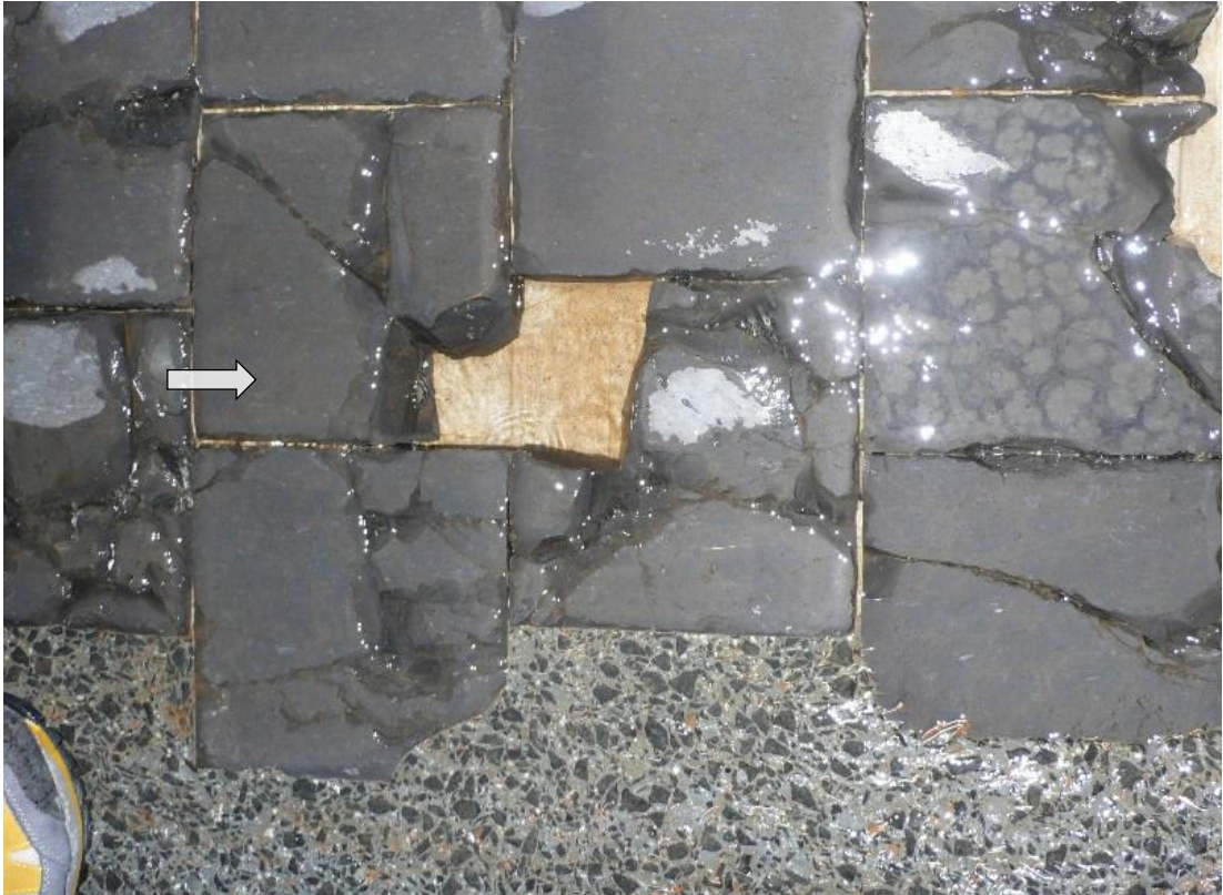
Figure 15: Damage in an area with cast basalt tile paving, picture taken 2012
