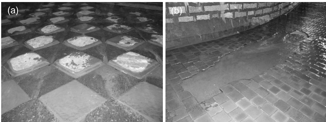
Figure 9: Abrasive wear in flow direction and local damage. (a) Diagonally checkered cast basalt tiles with mortar panels in between, (b) field of subsequently scoured and washed out cast basalt tiles
