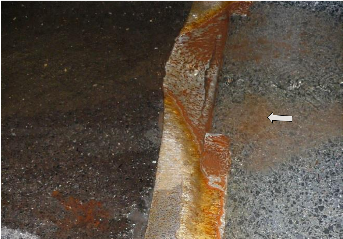
Figure 14: Damage on the steel beam separating the HPC field (right) from the SFC field (left), basaltic aggregates (dark grains) are visible, picture taken 2012
