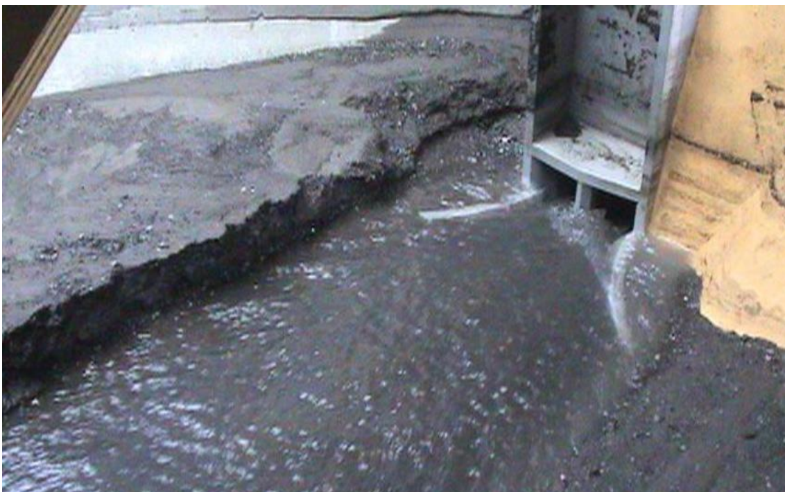
Figure 5: Residual deposits at the end of one of the hydro-sedimentary test
