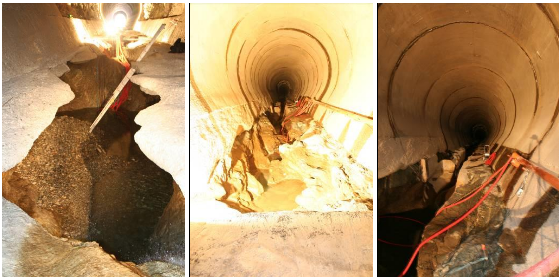
Figure 2: Eroded invert concrete and underlying Gneiss rock (2011)
