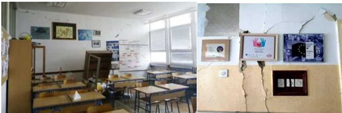
Figure 4.60. Earthquake damage in Glina High School (source: Facebook Page - Srednja škola Glina).
