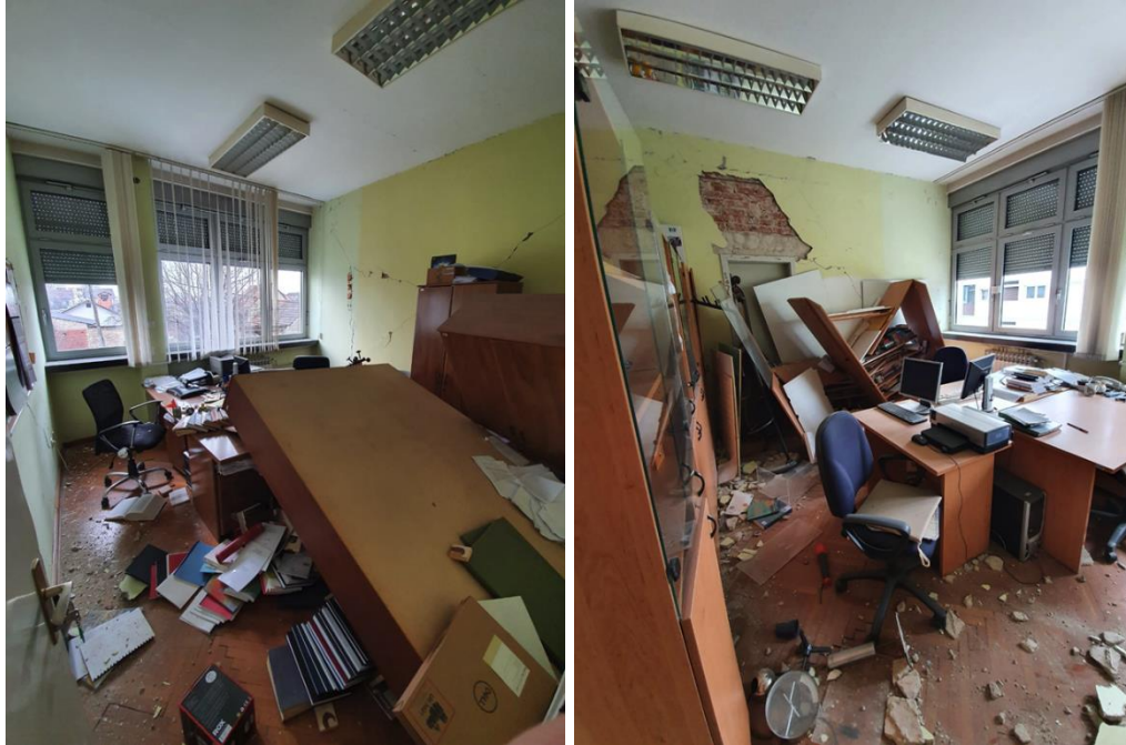
Figure 4.68. Diagonal cracks in infill walls and overturned shelves (source: Marko Bartolac).
