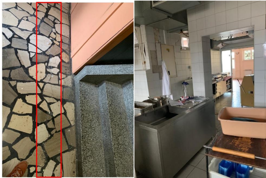
Figure 4.36. Cracks in the floor tiles (left) and tiles detached from the kitchen walls (right) (source: Damir Lazarević).
