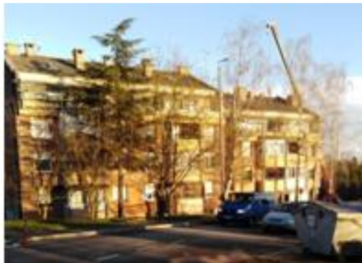
Figure 4.24. Removal of the chimneys from the roof of an RC building, "Brzaj" settlement in Sisak (source: Maja Freiberger).
