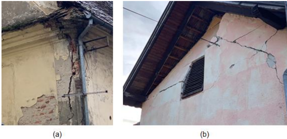
Figure 4.8. Out-of-plane damage of masonry walls: (a) vertical cracks (source: Damir Lazarević) and (b) cracking and onset of failure in gable walls (source: Nenad Bijelić).
