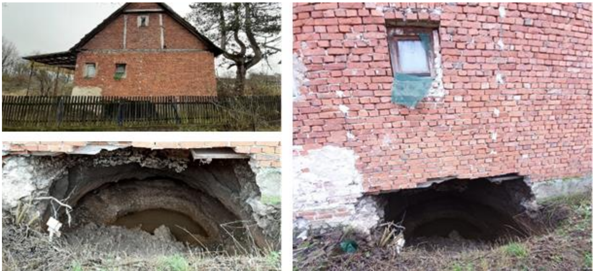
Figure 6.25. Sinkhole under a house with quite weak foundations (photos: left: Sonja Zlatović, right: Joško Krolo).
