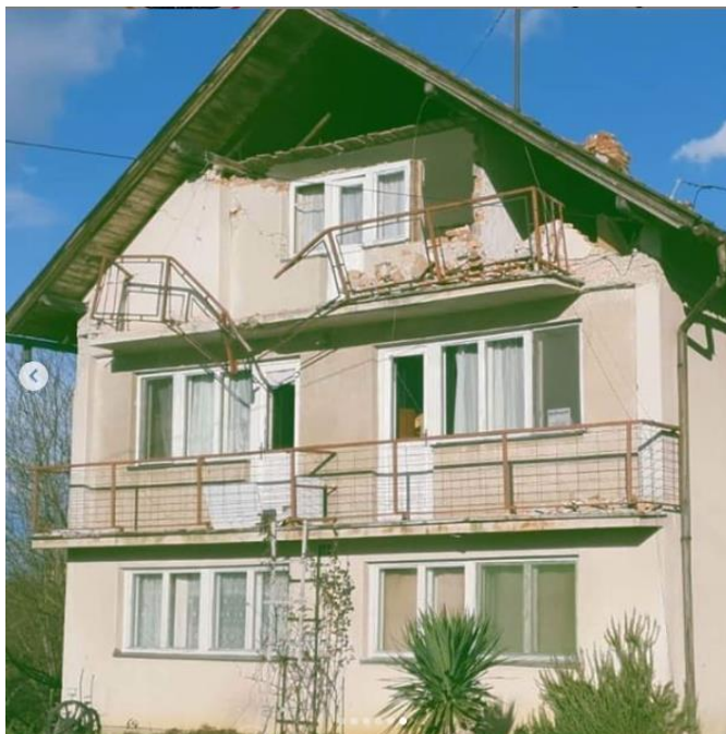
Figure 4.117. Damaged balcony guardrail in a family house in Sisak due to collapse of the gable end wall above (source: Instagram account on_a_binge_art).
