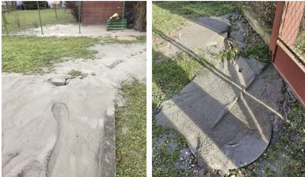
Figure 6.10. Liquefaction ejecta in Petrinja (Location: 45° 26' 38.6694"N, 16° 16' 33.5238"E, photo: Marko Bartolac).
