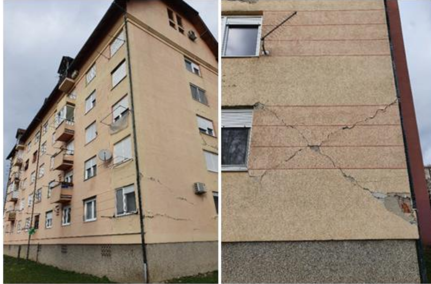
Figure 4.21. Damage to Building 4, a 5-story building with a vertical extension (source: Marko Bartolac).
