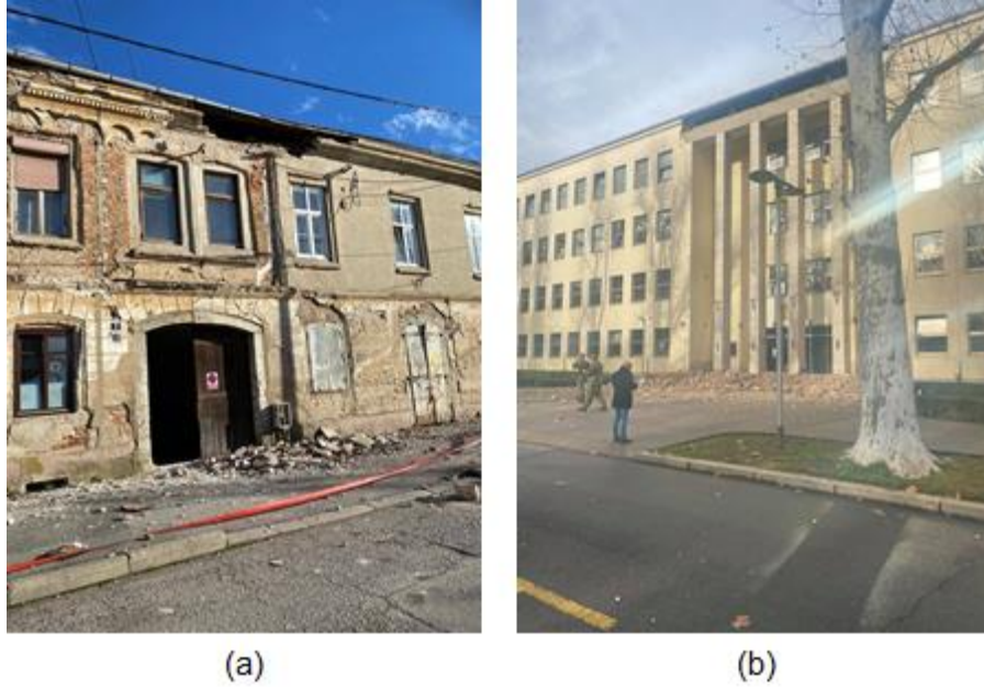
Figure 4.115. Fallen façades and parapets (source: 24sata.hr).
