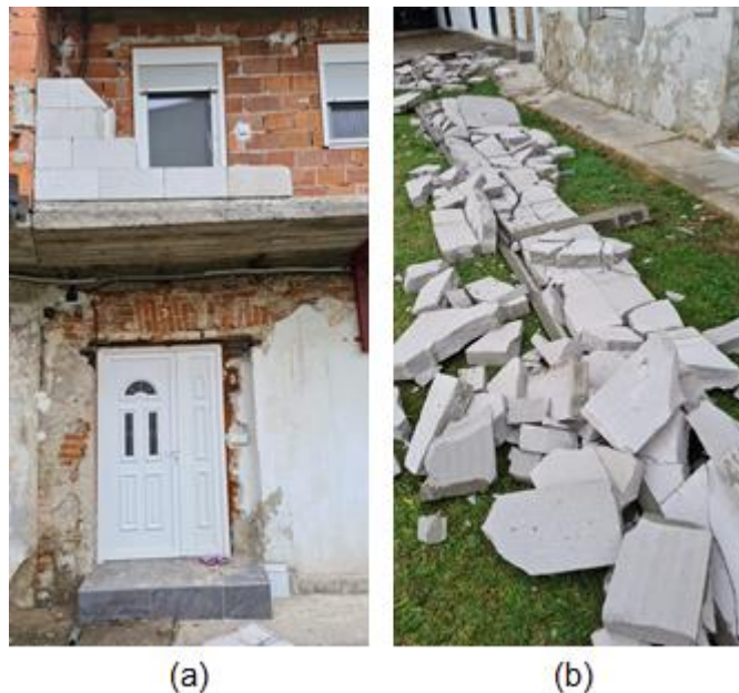
Figure 4.116. Collapsed unreinforced masonry balcony guardrail (source: Nenad Bijelić and Damir Lazarević).
