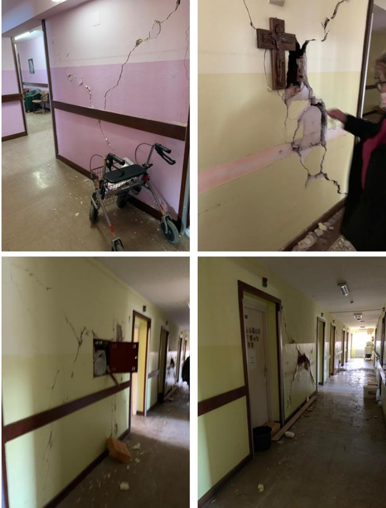
Figure 4.32. Damage to partition wall in the retirement home in Petrinja (source: Damir Lazarević).
