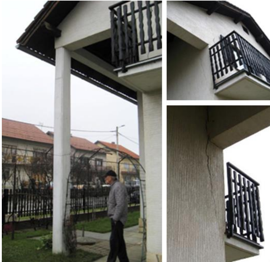
Figure 6.16. Liquefaction occurred under and around the residential building in the photograph. Sand appeared just next to the house, along the fence, and the area covered with bricks moved up. Cracks opened as the house sank. Petrinja, Ulica Vilima Muhe (45.43514, 16.2684, source: Sonja Zlatović).
