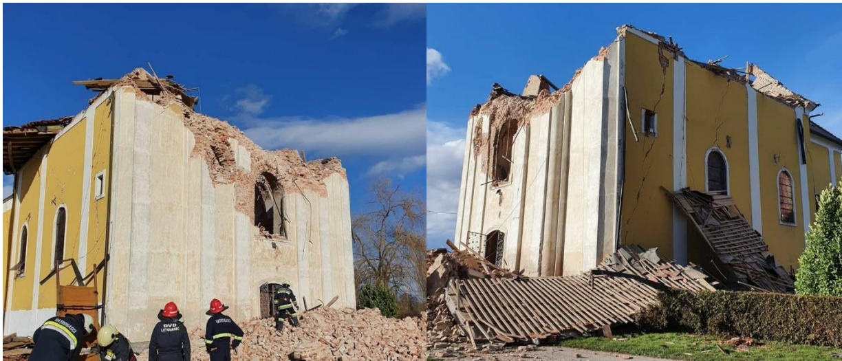
Figure 4.92. Church of St. Nikola and Vid in the village of Žažina after it suffered the collapse of a campanile and roof structure (source: Instagram account visitlekenik).
