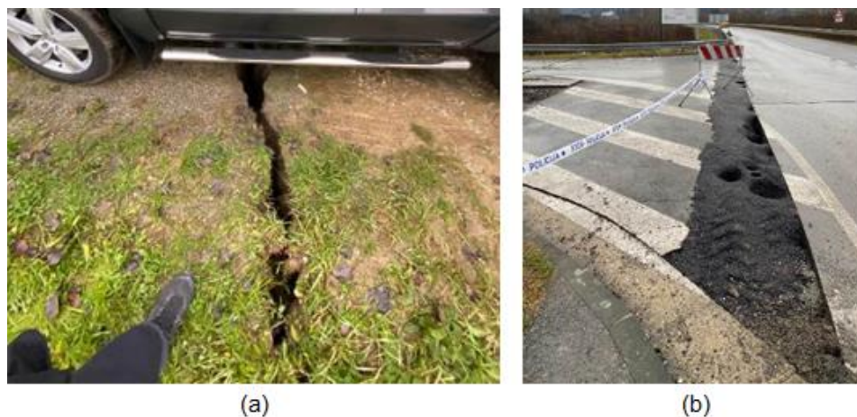
Figures 5.8. (a) Wide cracks at the bridge embankment and (b) collapsed portion of the asphalt curtain at the intersection with the access road to the center of Petrinja (source: Mate Baričević).
