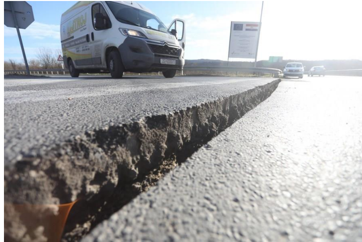
Figure 5.14. A major fissure in the road in Sisak was observed after the December 29, 2020 earthquake (source: Marin Tironi/Pixsell via Xinhua).
