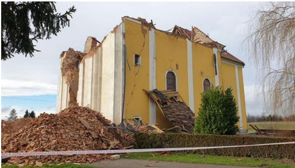
Figure 4.90 Church of St. Nikola and Vida in the village of Žažina after the earthquake exhibited severe collapse of the bell tower and extensive cracking of load bearing walls (source: Total Croatia News 2021).
