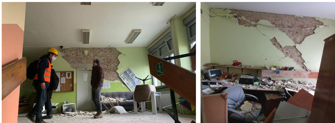
Figure 4.67. Plaster detached from the wall (source: Damir Lazarević and Marko Bartolac).
