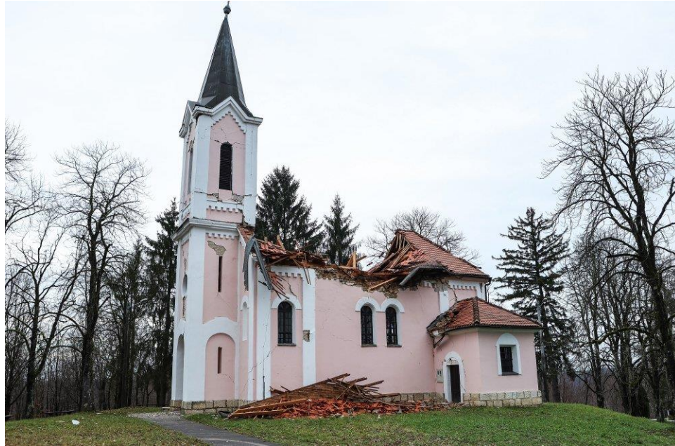
Figure 4.102. Church in Mračaj, near village Majur. Collapse of the timber roof structure and cover and severe cracking of the bell tower (source: Marko Pripic/PIXSELL).
