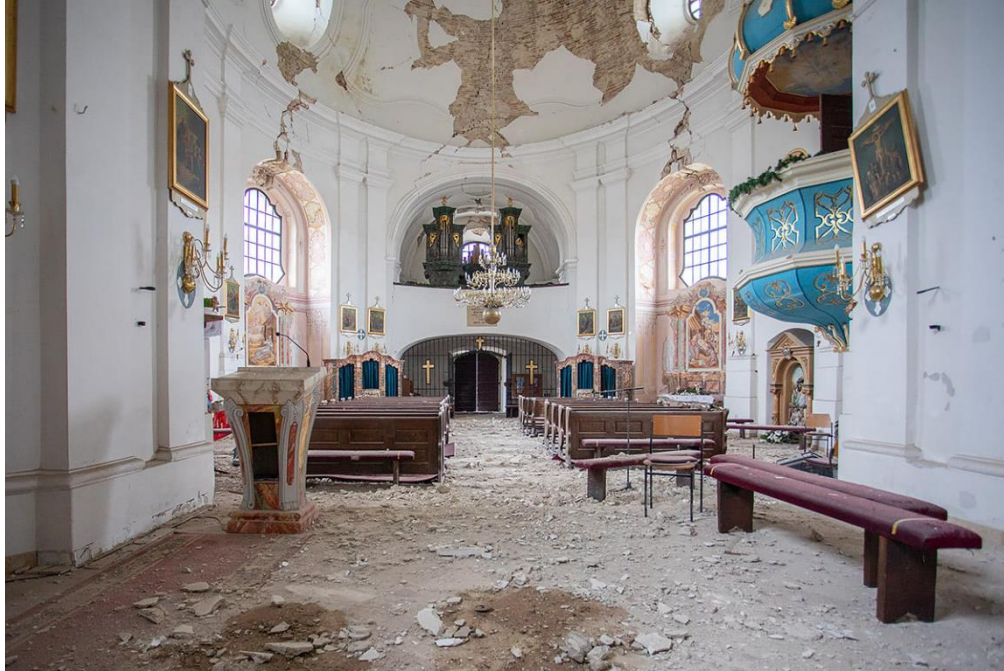
Figure 4.94. Interior of the Church of St. Marije Magdalene in Sela. Extensive cracking visible in the dome, as well as plaster detachment (source: Facebook Page Sisačka biskupija).
