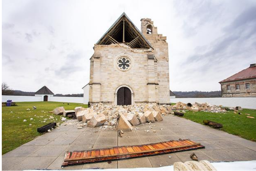
Figure 4.95. Church of Our Lady of the Mountain in the village Gora after its triangular gable suffered out-of-plane failure and the part of the bell tower collapsed (source: Facebook Page - Sisačka biskupija).
