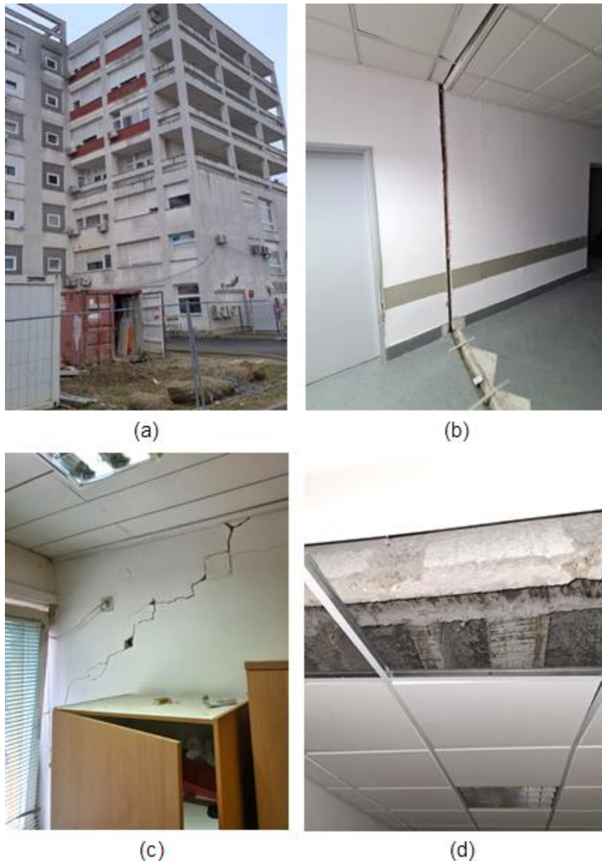
Figure 4.44. Building #5: (a) Outside view, (b) joint opening, (c) concrete wall cracking, and (d) fallen ceiling tiles (source: Nenad Bijelić).
