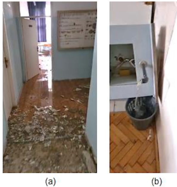
Figure 4.49. Leaking water pipe in the First Primary School in Petrinja: (a) water on the floor and (b) broken water pipe (source: Nenad Bijelić).
