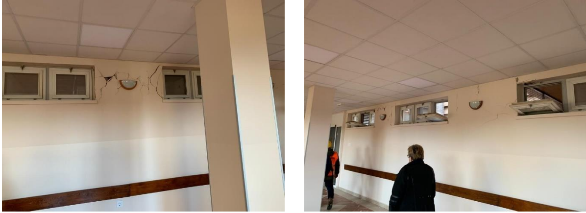
Figure 4.31. Shear cracks in infill masonry walls of the retirement home in Petrinja (source: Damir Lazarević).
