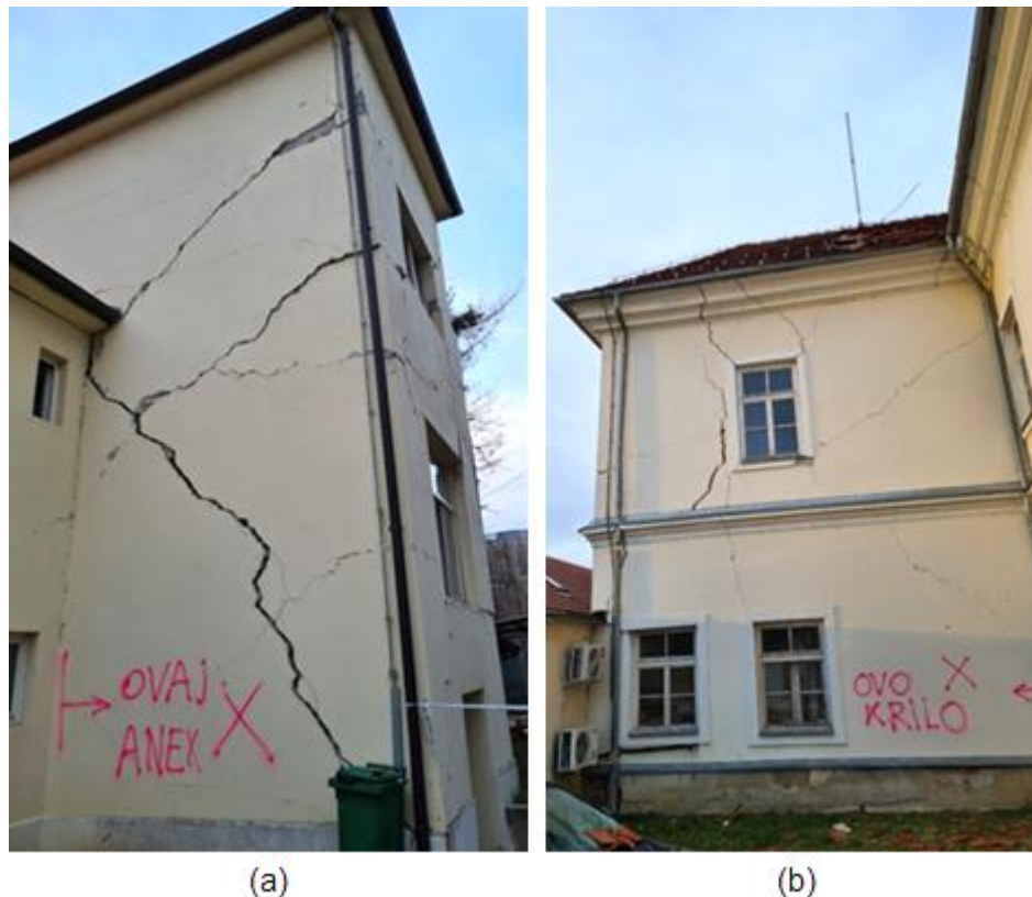
Figure 4.79. Town hall annexes after the earthquake: (a) Southwestern annex with widespread damage in the transverse wall (source: Nenad Bijelić) and (b) Northwestern annex with the widespread damage in the transverse wall (source: Nenad Bijelić).
