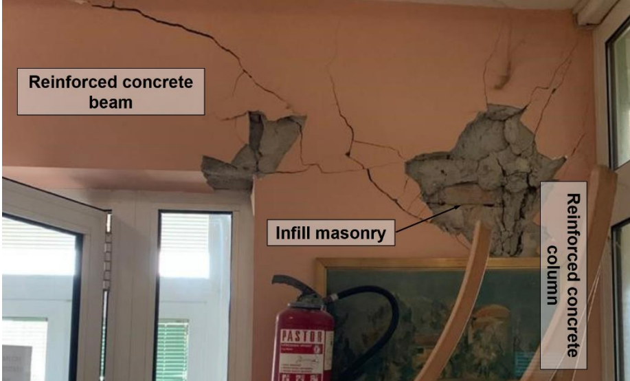
Figure 4.34. Damage to a reinforced concrete beam in the retirement home in Petrinja (source: Damir Lazarević).
