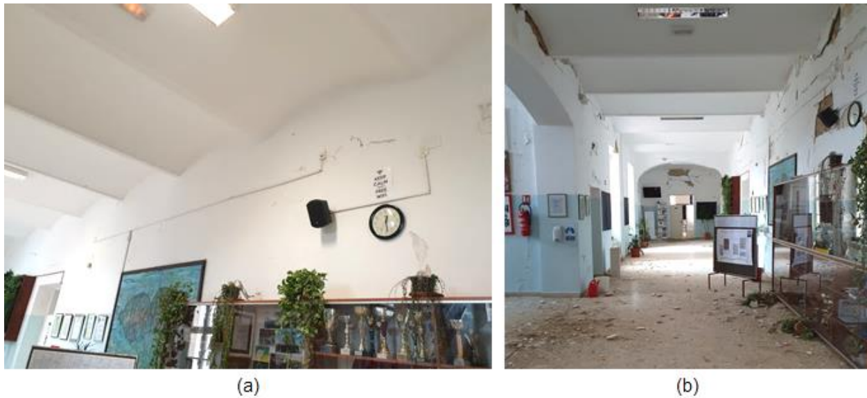
Figure 4.53. Interior of Petrinja High School: (a) minor damage caused by the December 28 earthquake (source: Domagoj Damjanović) and (b) significant damage caused by the December 29 earthquake (source: Marko Bartolac and Nenad Bijelić).
