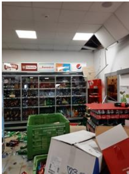
Figure 4.27. Damage to hung ceiling assembly in the KTC supermarket (source: Sonja Belovarac Radenovic).
