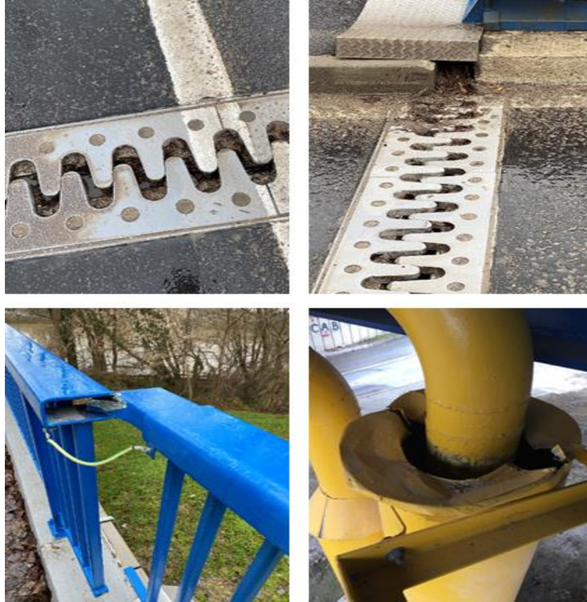
Figure 5.12. Damage due to lateral displacement of the bridge relative to the slab approach, Galdovo Bridge (source: Mate Baričević).
