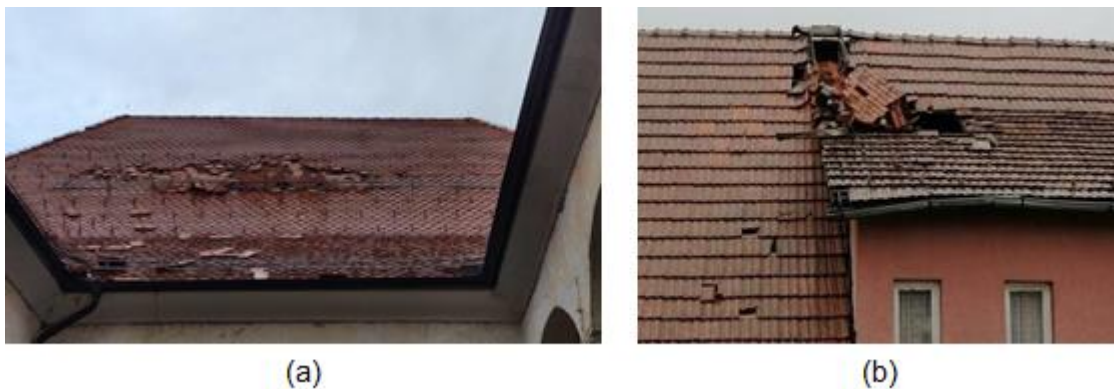
Figure 4.122. Damaged roof tiles (source: rtvslo.si).
