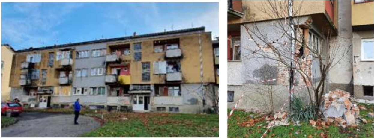
Figure 4.16. Damage in a 3-story residential building in Petrinja (source: Marko Bartolac).
