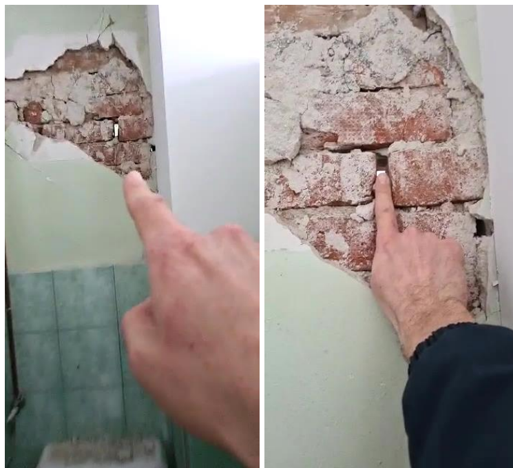
Figure 4.71. Gapping in head joints of infill walls (source: Nenad Bijelić).
