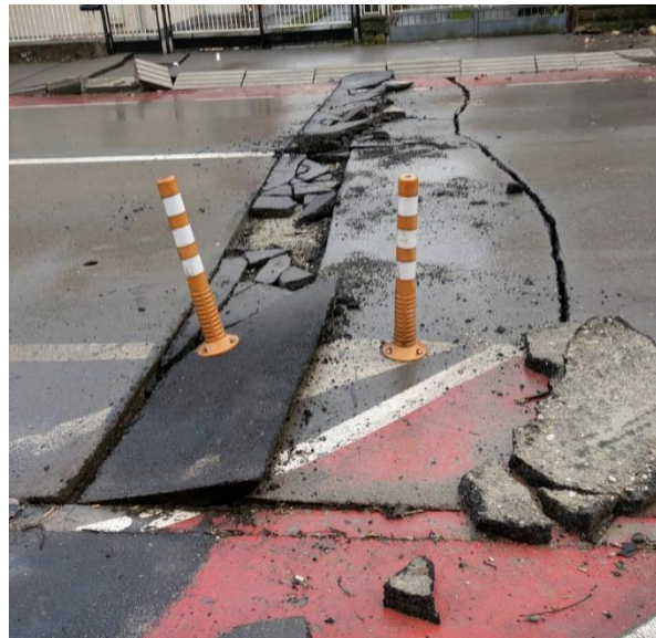
Figure 6.23. Road pavement cracking (45°29'45.108"N,16°22'36.888"E, source Zeljko Arbanas).
