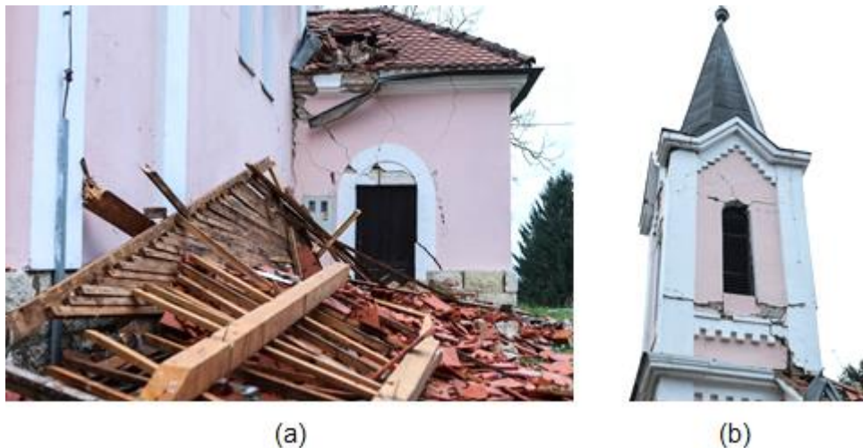
Figure 4.103. Church in Mračaj, near village Majur: (a) heavy cracking in the interface between adjacent shorter unit and the main nave (source: Marko Pripic/PIXSELL) and (b) severe cracking of the bell tower (source: Marko Pripic/PIXSELL).
