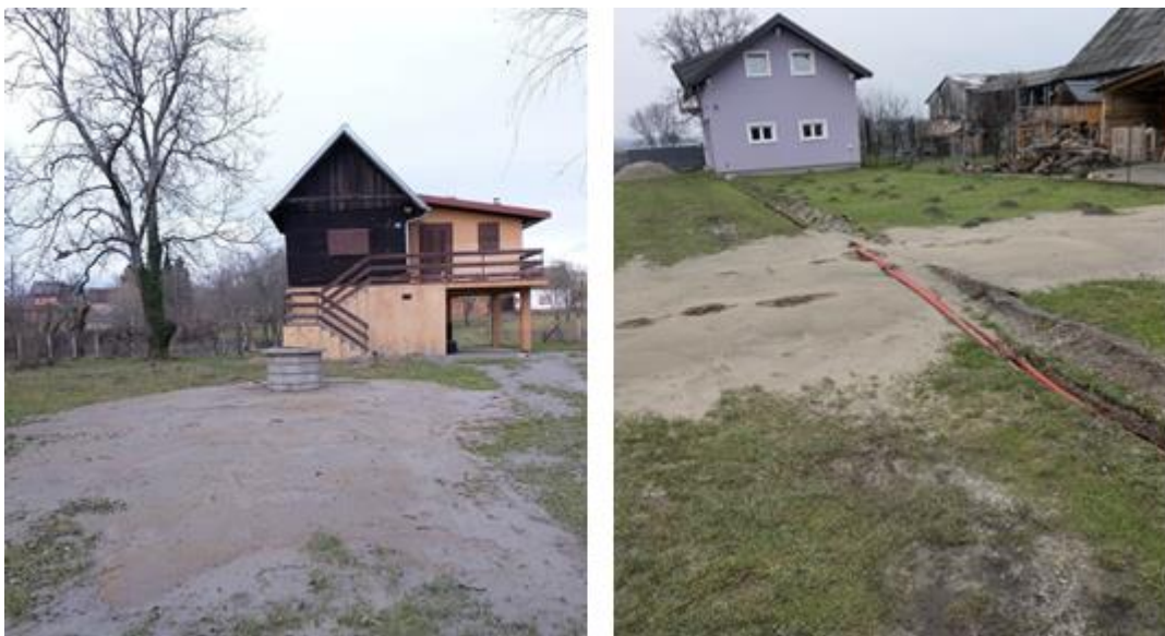
Figure 6.12. Liquefaction surface manifestation and floatation of manholes in Petrinja (left: 45° 29' 5.25"N, 16° 9' 52.306"E; right: 45° 31' 10.986"N, 16° 24' 16.416"E; source: Željko Arbanas).
