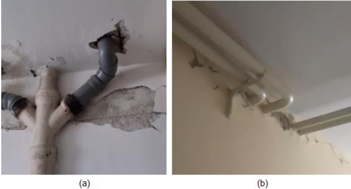
Figure 4.114. Examples of failures in piping systems in university building constructed in 1962 (Uciteljski fakultet) (source: Nenad Bijelić and Damir Lazarević).
