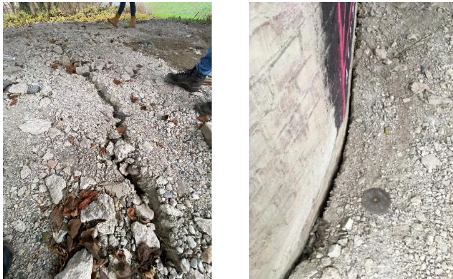
Figure 5.13. The displacement of the platform is visible on the ground, Galdovo Bridge (source: Mate Baričević).
