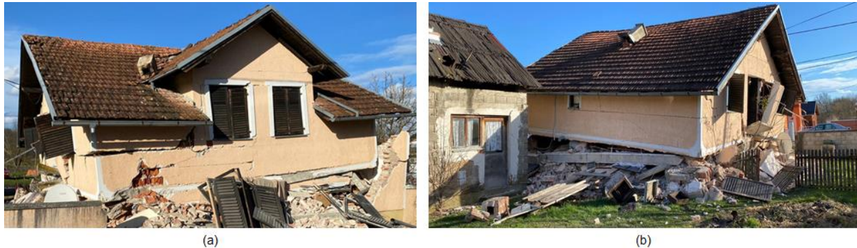
Figure 4.14. Collapsed partially confined masonry building in Prekope village, close to Glina (sources: (a) Damir Sencar AFP Getty and (b) Krešimir Micić).
