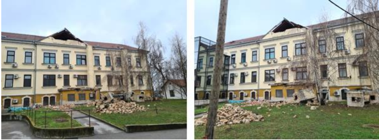
Figure 4.119. Fallen chimneys and gable end wall in hospital Dr. Ivo Pedišić in Sisak (source: Nenad Bijelić and Marko Bartolac).
