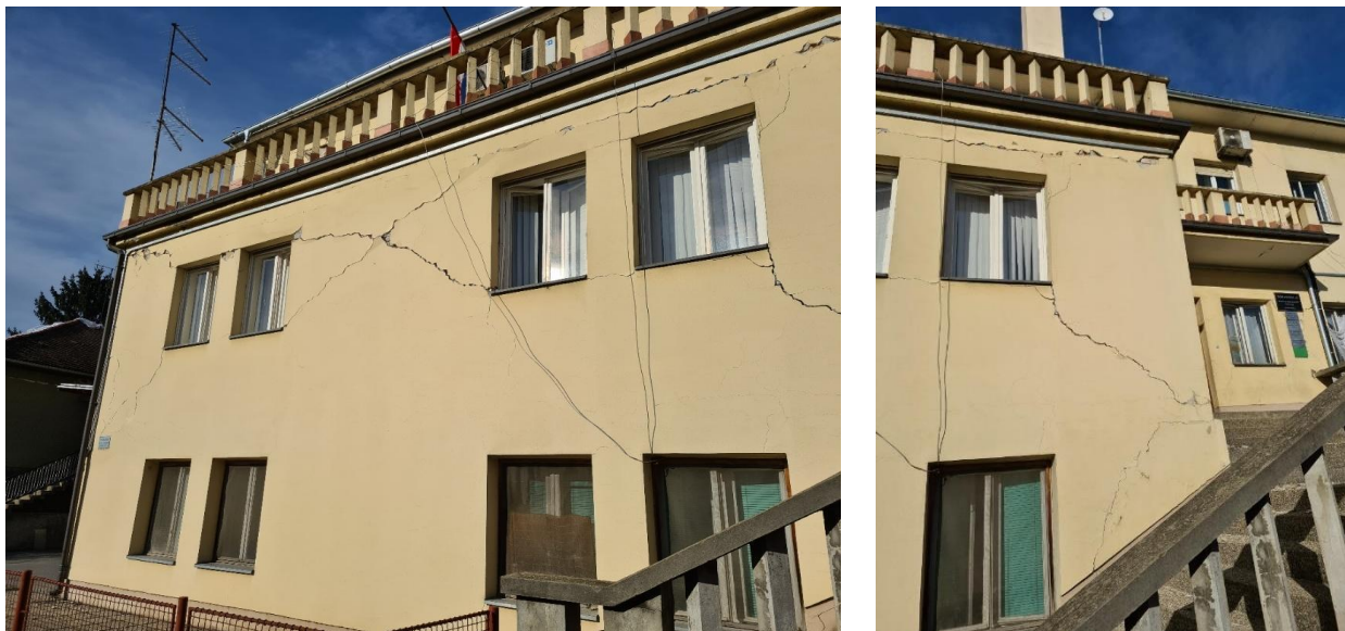
Figure 4.38. Photos showing the exterior of the health center in Petrinja with large shear cracks in the exterior walls (source: Domagoj Damjanović).
