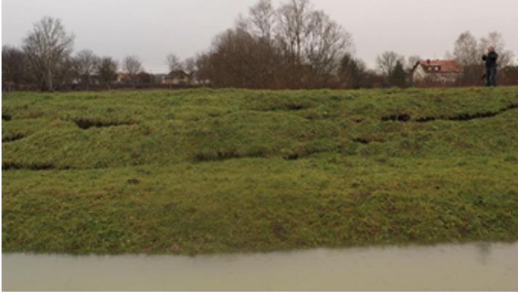
Figure 6.15. Embankment failure of river Sava near Hrastelnica (source: Croatian Waters Archive).
