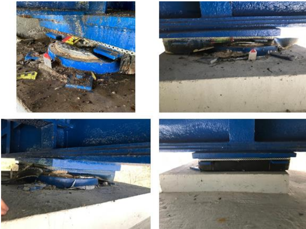
Figure 5.11. Rubber bearings at the abutments failed due to relative displacement demands between the support and the superstructure exceeding the capacity of the bearings, Galdovo Bridge (source: Mate Baričević).
