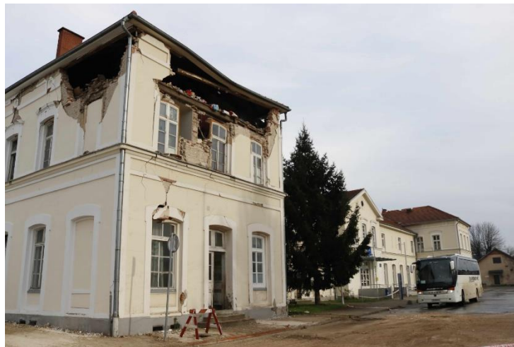
Figure 5.4. Significant damage of the Sisak Railway Station building (source: CroatiaWeek).
