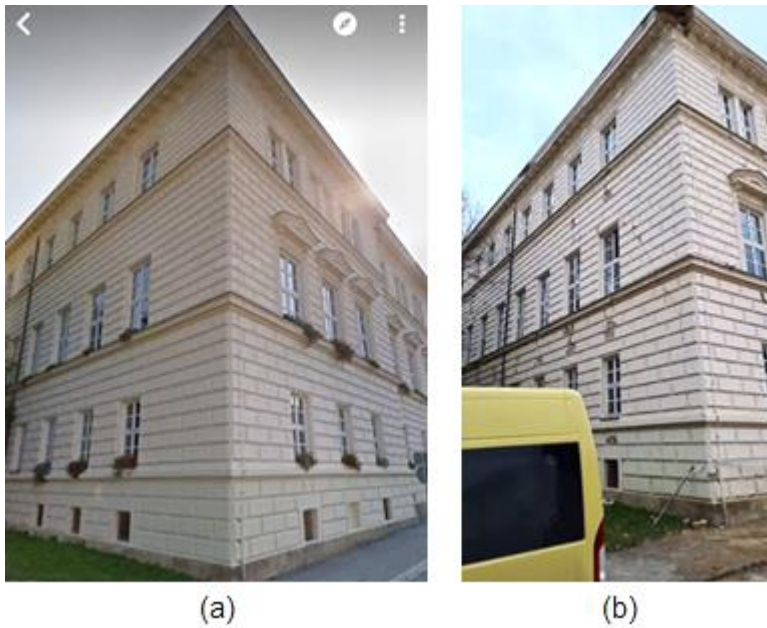
Figure 4.51. Transverse wall of Petrinja High School (a) before the earthquake (source: Google Street View) and (b) after the earthquake (source: Nenad Bijelić).
