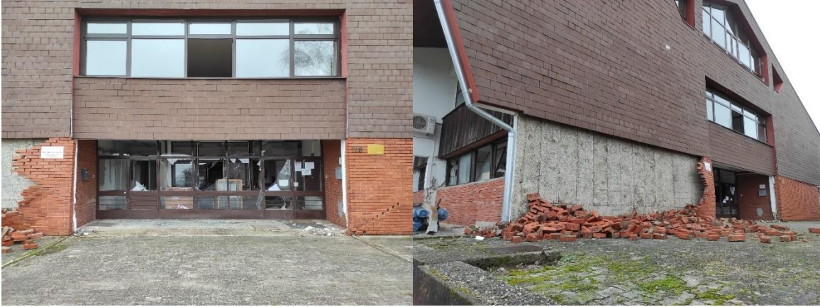
Figure 4.63. Brick facade detached from building (source: Nina Čeh).
