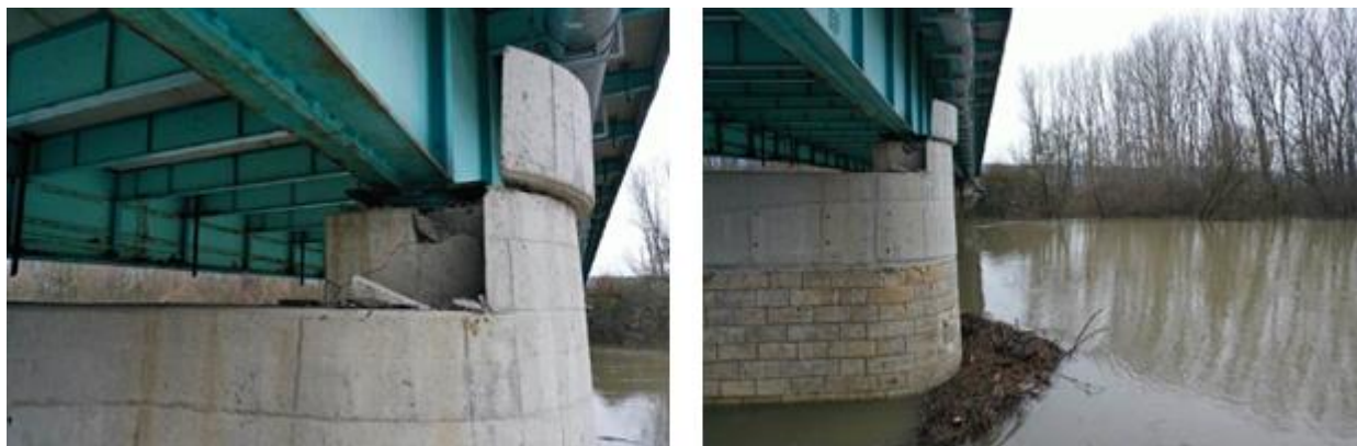
Figure 5.6. Damaged bearing supports of the Brest Bridge (source: Mate Baričević).
