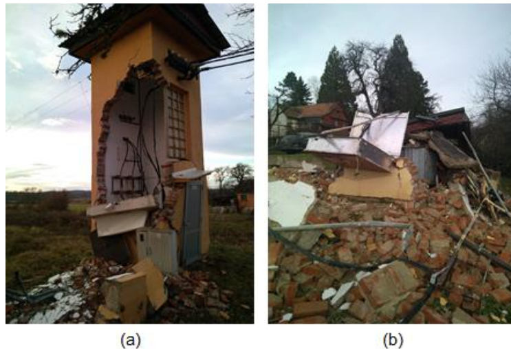
Figure 5.2. Severely damaged (a) and collapsed (b) substations in the Petrinja area. The size of substation structure on the left is 2.5 m square in plan and 8 m high (source: Mladen Štajdohar).
