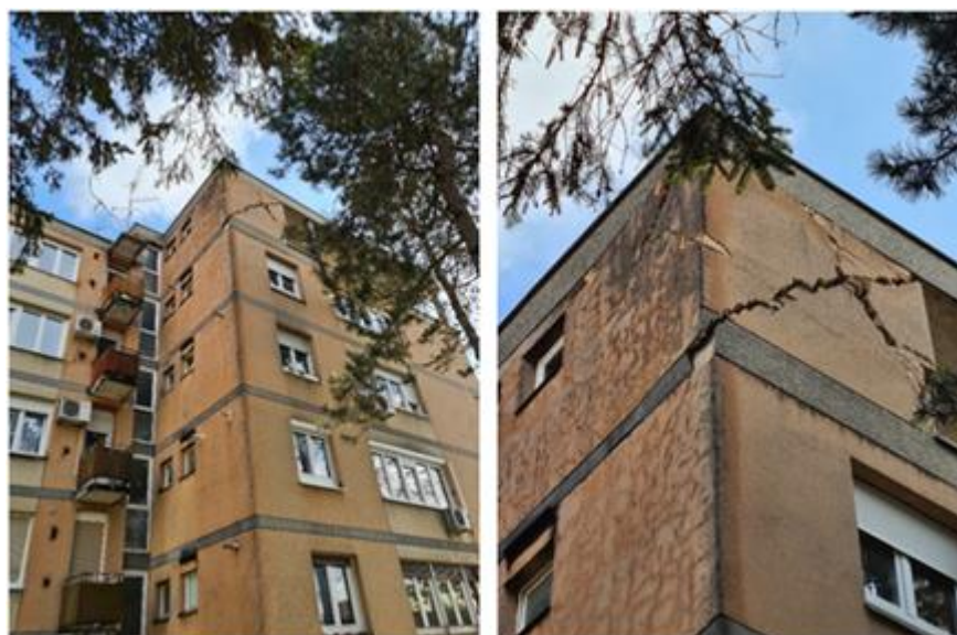
Figure 4.20. Extensive cracking experienced at the roof/terrace level of Building 2 (source: Nenad Bijelić).
