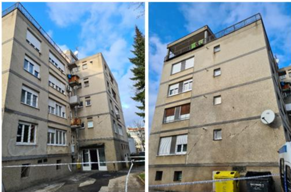
Figure 4.19. Damaged Building 3: exterior view and cracking pattern at the ground floor level (source: Nenad Bijelić).
