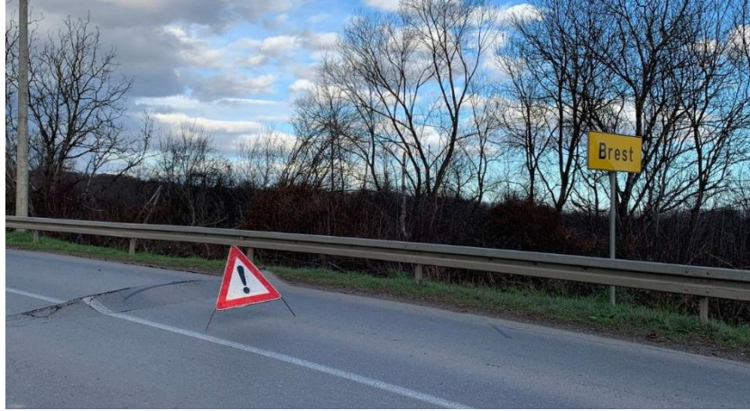
Figure 5.16. Ground failure of the road close to the Brest Bridge (source: Index.hr 2020d).
