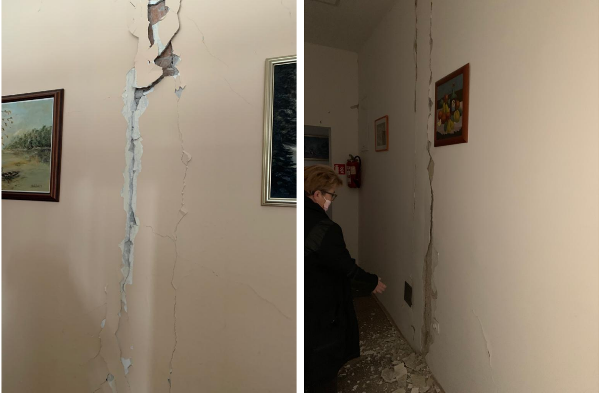
Figure 4.33. Cracks along the interface between a masonry infill and an RC column (source: Damir Lazarević).
