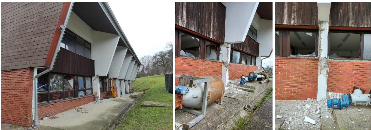
Figure 4.65. Shear cracks to exterior RC columns (source: Nina Čeh).
