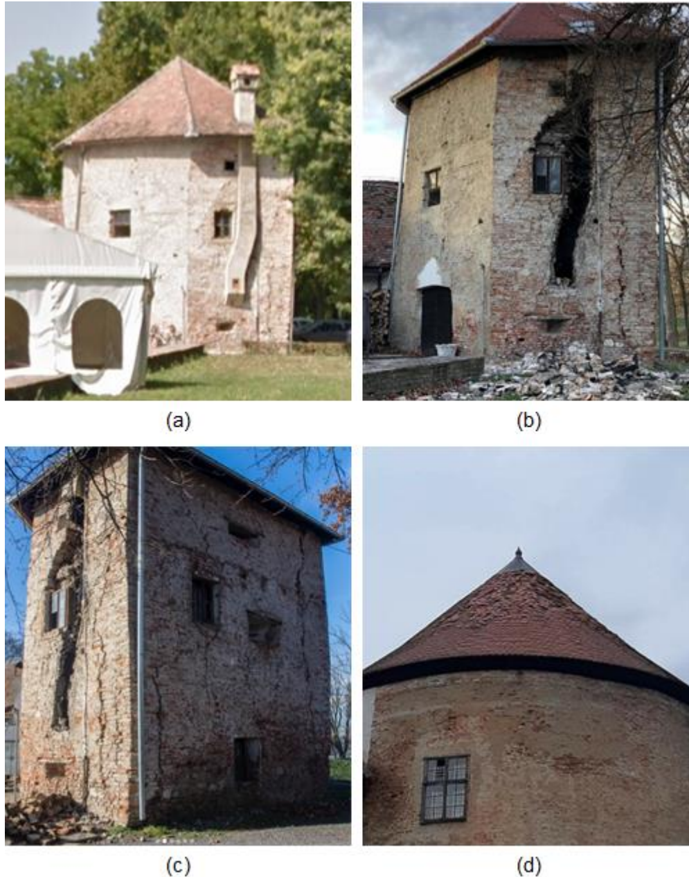
Figure 4.83. (a) Small tower connected to the Sisak fortress in 2011 (source: Google), (b, c) collapsed chimney in the small tower, and (d) damage to the tiles of the conical roof of one of the tower of the fortress (source: Instagram account starigradsisak and dvorcistarigardovi).
