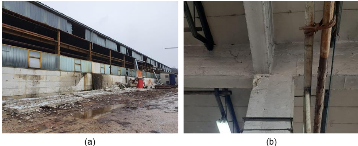
Figure 4.108. Damage to exterior cladding and concrete columns in an industrial facility in Sisačka ul. 116, 44250, Petrinja (source: Marko Bartolac).
