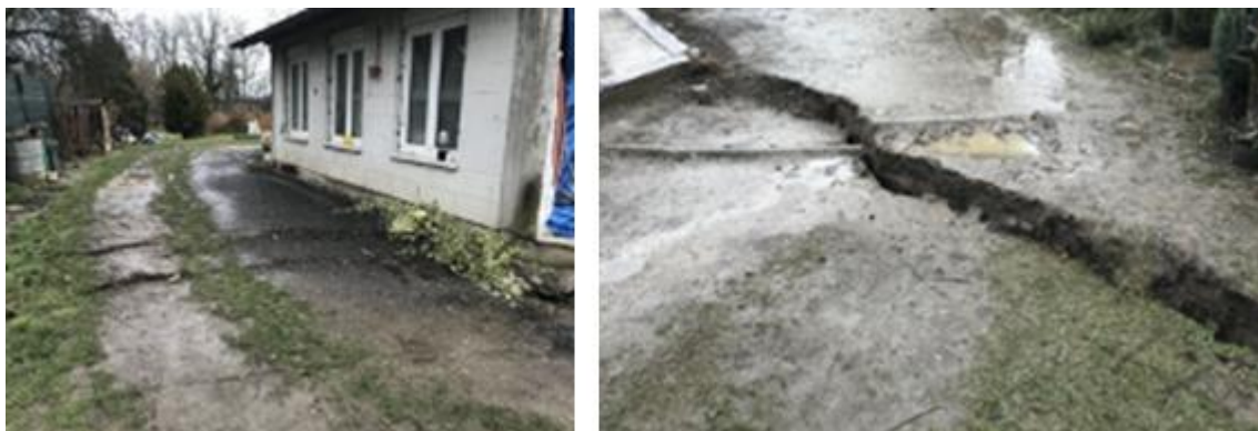
Figure 6.17. Building settlement due to lateral spreading, Bok Palanječki (photo: Vedran Jagodnik, 45°30'36.21"N,16°24'38.892"E).
