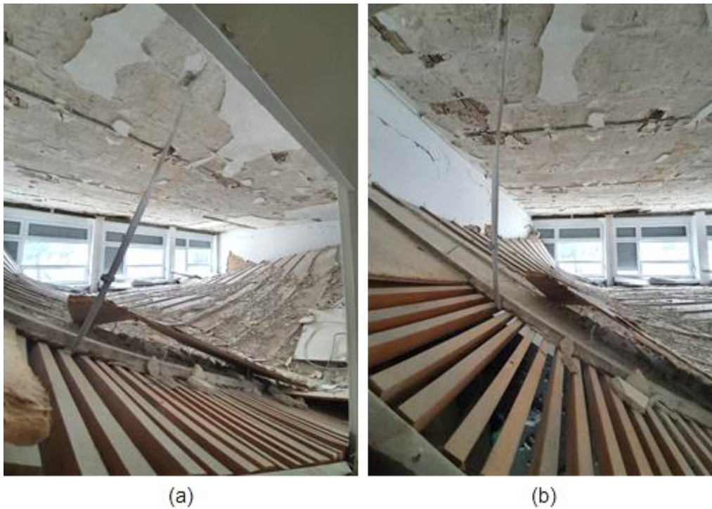
Figure 4.110. Ceiling collapse in 1962 university building (Učiteljski fakultet) (source: Marko Bartolac).
