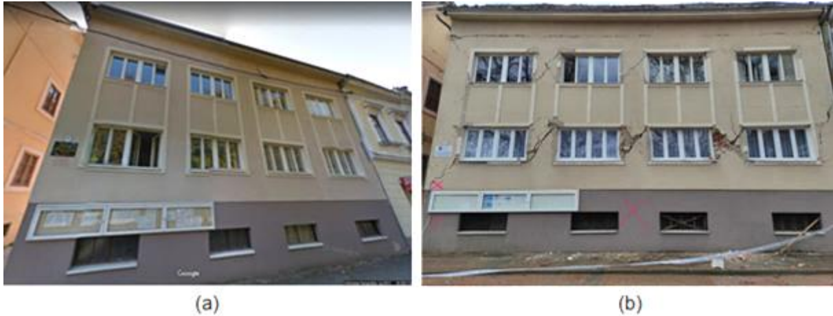
Figure 4.80. Chamber of Crafts building: (a) before the earthquakes (source: Google Maps) and (b) after the earthquakes. All central piers developed deep in-plane shear cracks. A wide continuous horizontal crack extends throughout the façade at the roof level (source: Nina Čeh).
