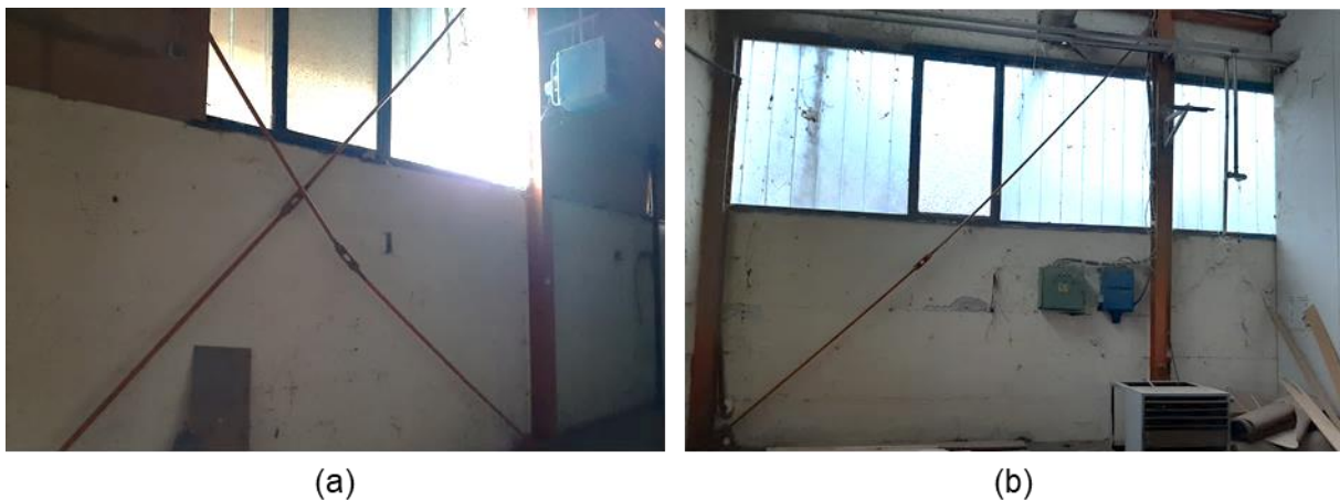
Figure 4.107. Fracture of tension-only steel bracings in an industrial facility in Sisačka ul. 116, 44250, Petrinja (source: Marko Bartolac).
