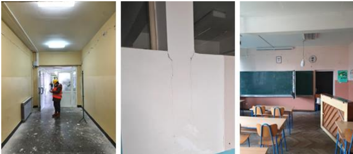
Figure 4.56. Cracks forming at the contact between reinforced concrete frames and masonry infills (source: Nenad Bijelić and Damir Lazarević).
