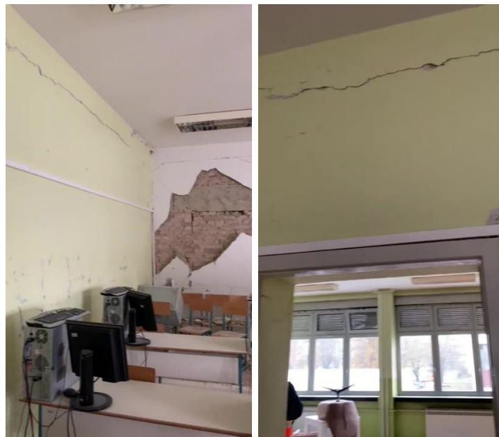
Figure 4.69. Horizontal cracks between the RC beams and the top of infill walls (source: Damir Lazarević).
