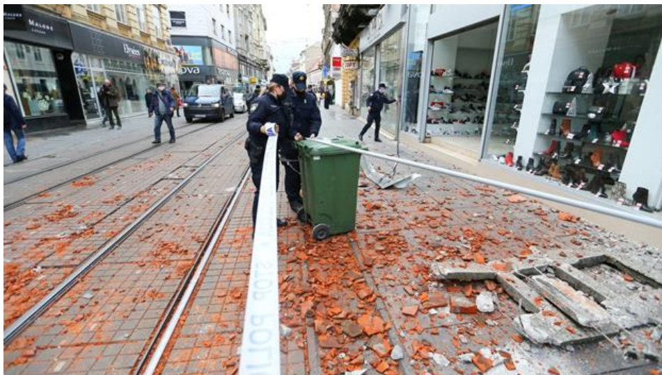
Figure 4.25. Photo taken looking east on Ilica Street in Zagreb showing fallen debris (source: Santora and Orovic, 2020).
