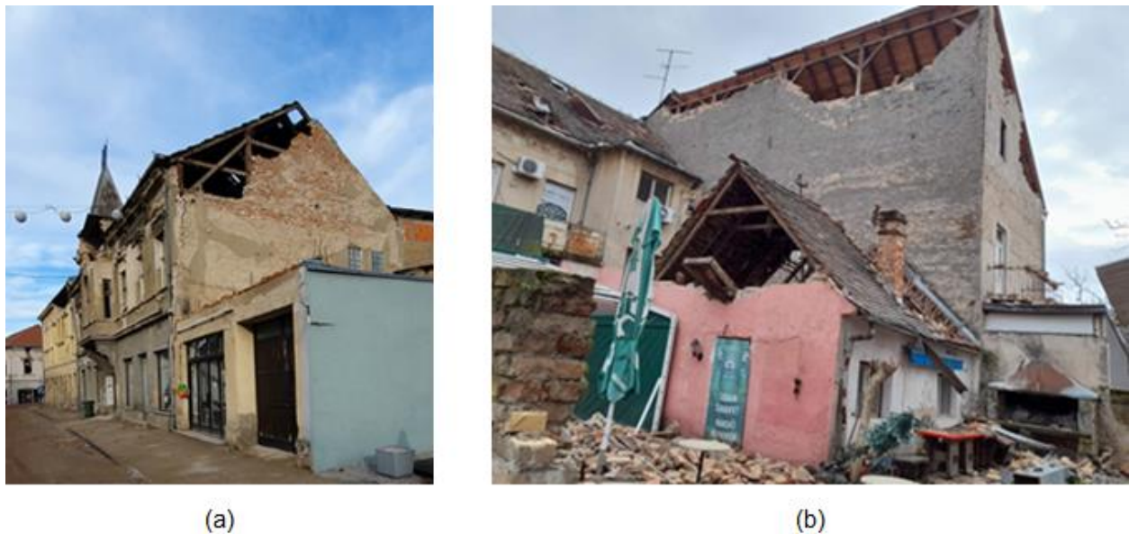
Figure 4.7. Out-of-plane failure of walls at the upper portion of buildings with wooden floors and roofs due to flexible diaphragm and the absence of adequate wall-to-floor connections: (a) older 2-story URM building in downtown Petrinja (source: Nenad Bijelić) and (b) rear wall of a 2-story building in Sisak (source: Kristijan Freiberger).
