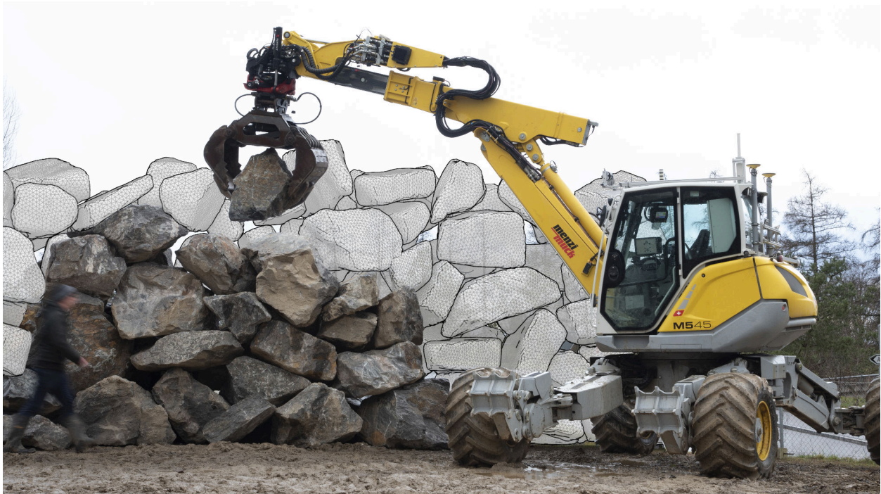
Figure 12: The presented mapping and manipulation tools in this paper were used for the application of dry stone wall construction with the autonomous hydraulic excavator HEAP. The in-progress wall is overlaid with a potential extension of the structure, generated by allowing the geometric planning to continue with additional digital stone models. Further details on the geometric planning of the desired stone poses can be found in (Johns et al., 2020).
