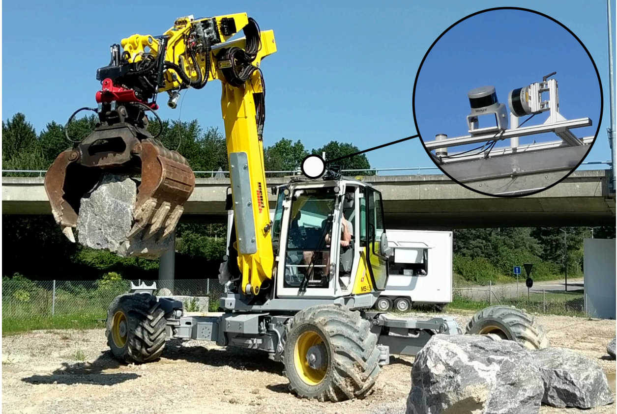
Figure 2: HEAP is an autonomous walking excavator based on a highly customized Menzi Muck M545. It is equipped with onboard sensors for state estimation (GNSS, IMUs, and encoders) and scanning the environment (3D LiDARs). As shown in the inset, the two LiDARs are mounted perpendicularly to each other such that a scanning motion is achieved not only while driving the robot around, but also while swinging the cabin.
