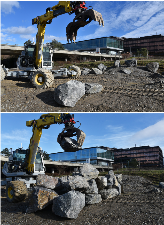
Fig. 10 Wall construction in progress with two (above) and twenty (below) placed stones out of the 40 used in this experiment.
