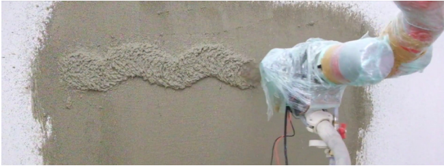
Fig. 7: First results in robotic plastering. The robot applies plaster on the wall with a spraying nozzle.
