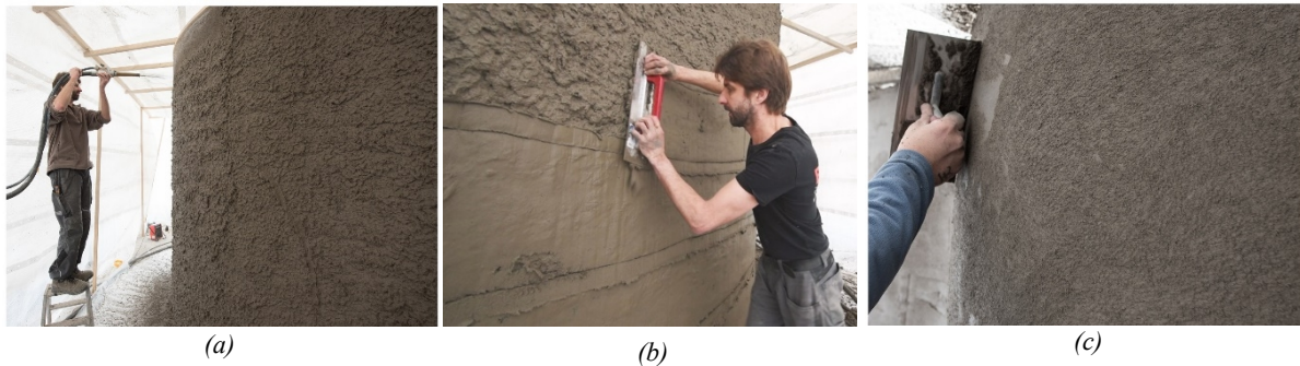
Fig. 24: Surface finish process: (a) applying a layer of shotcrete; (b) distributing the material using a modified trowel with distancers; (c) scraping off excess material.
