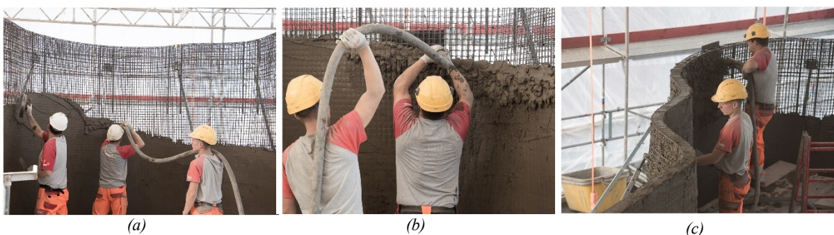
Fig. 23: Filling process: (a) trowelling the freshly filled mesh; (b) close-up of the filling process showing the un-trowelled concrete; (c) filling the upper region of the mesh.
