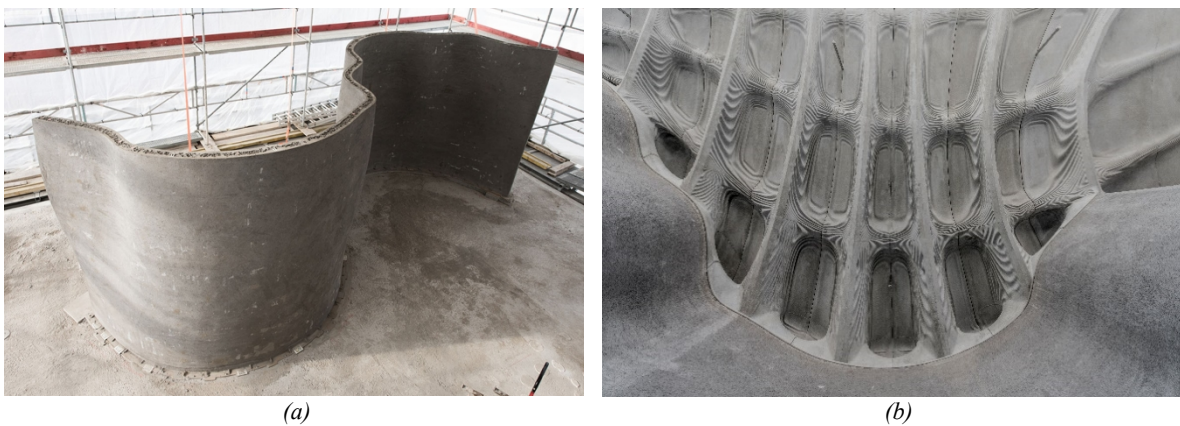
Fig. 26: Mesh Mould wall: (a) after the cover layer was applied (b) after installation of the Smart Slab.
