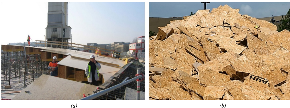
Fig. 2: EPFL Rolex Learning Center construction process: (a) installation of the unique formwork tables; (b) construction waste after stripping the formwork.
