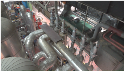
(a) Complex industrial environment used in our aerial teach-and-repeat inspection demonstrator [29]. Video: https://goo.gl/LoNz1j
