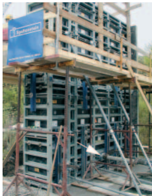
Fig. 1: Formwork used for the field study with a valve located at its base (pointer).
