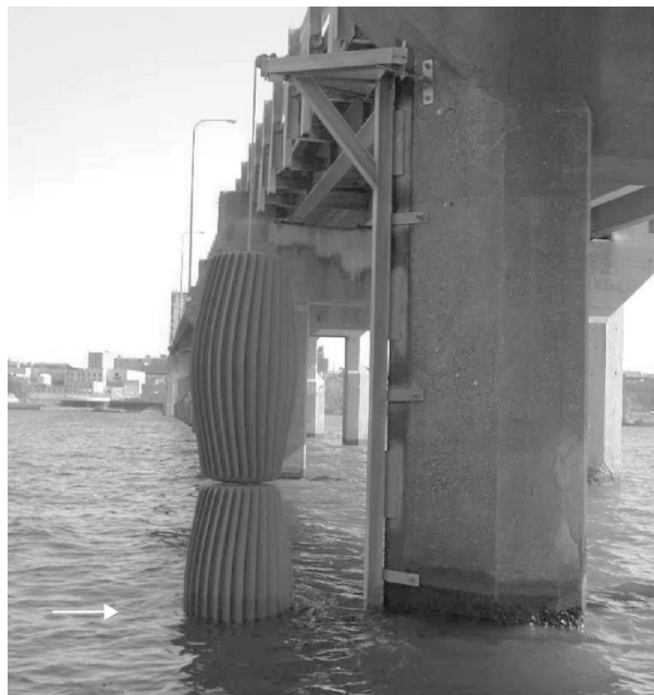
Figure 3.13 Double-stacked installation of a LW sweeper at the Mississippi River, USA (adapted from Bradley et al. 2005)
