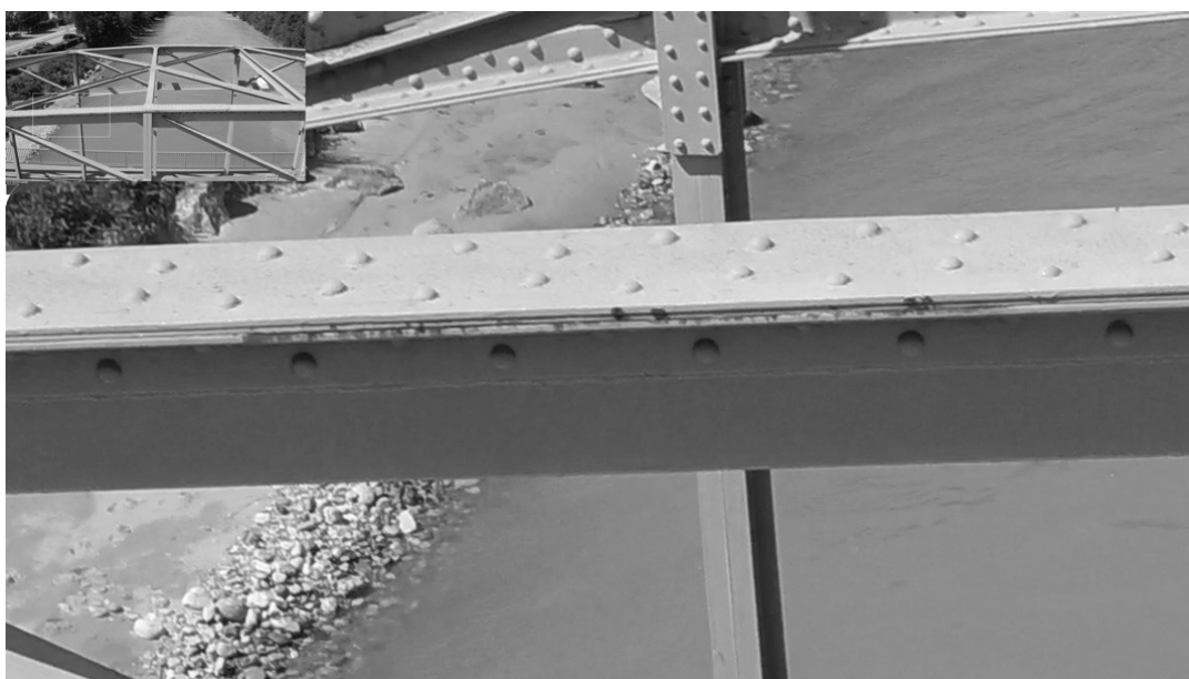
Figure 3. Corrosion marks on steel girder, magnified from top left hi-res image.
