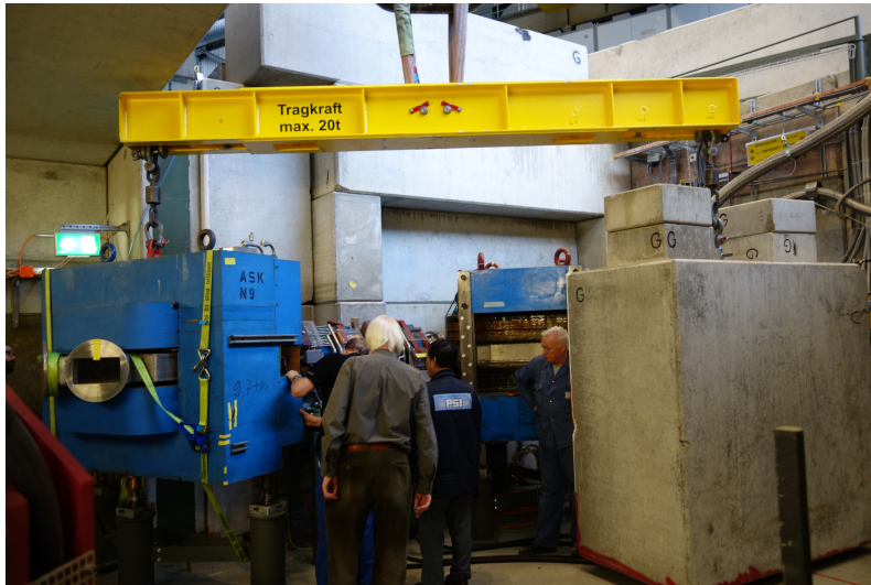
Figure 2.48.: By attaching the ASK dipole magnet to a steel beam with a 10 ton concrete block as a counterweight, the ASK could be accurately placed below the \pi E3 area floor.
