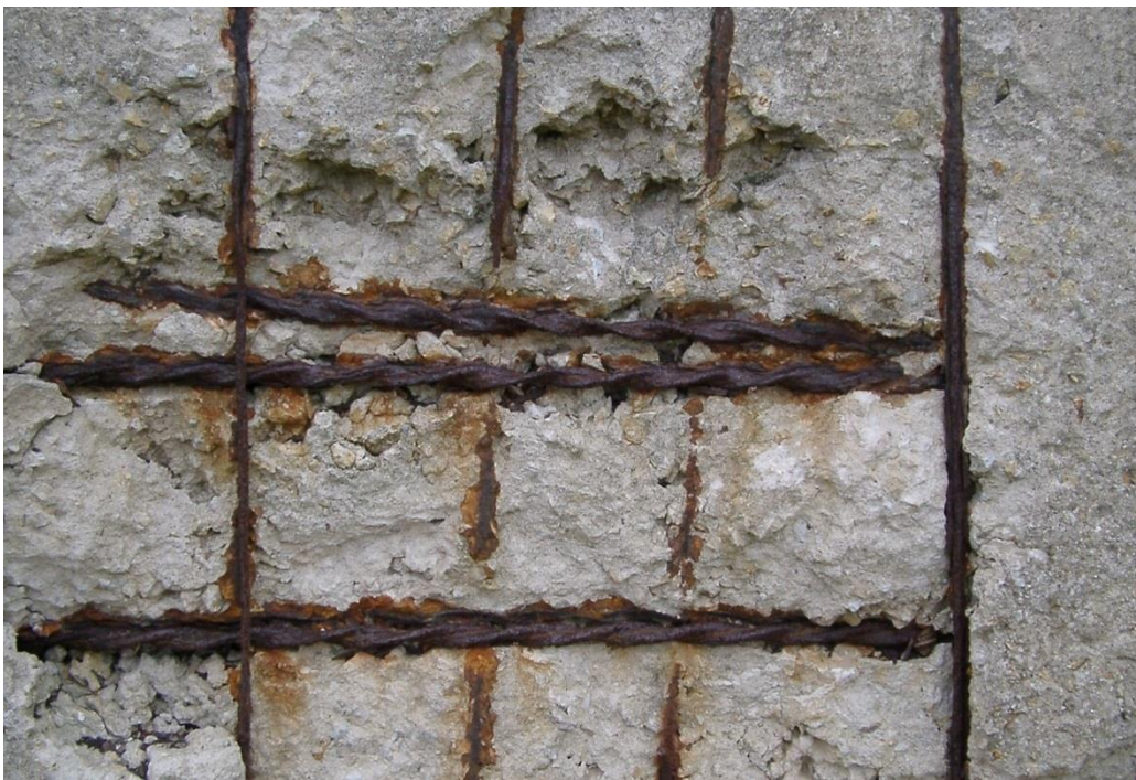
Fig. 19 Corroded reinforcements in a section of concrete beam (Bertolini, Elsener et al. 2013)
