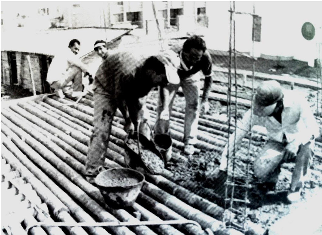
Fig. 36 Bamboo culms used as reinforcement and providing voids for concrete floor in Colombia (Hidalgo-Lopez 2003)
