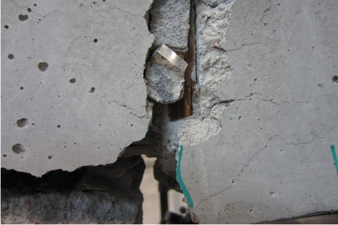
Fig. 163 Failure of the steel cable ties used to hold the vertical legs of the stirrups
