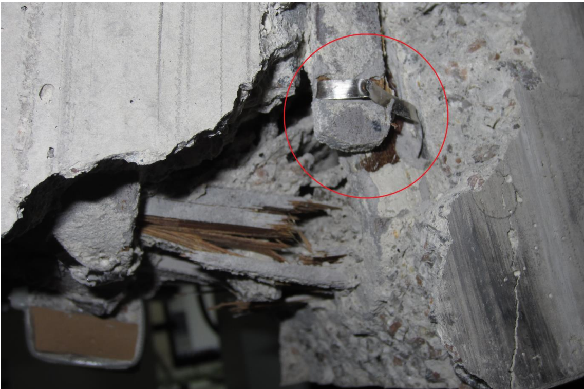
Fig. 164 The opening of the steel cable ties followed by the ultimate failure of the beam
