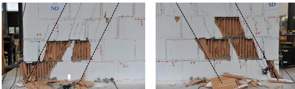
Figure 4-9. Final crack pattern at the base of a flexure-dominated URM wall (Wall T7)
