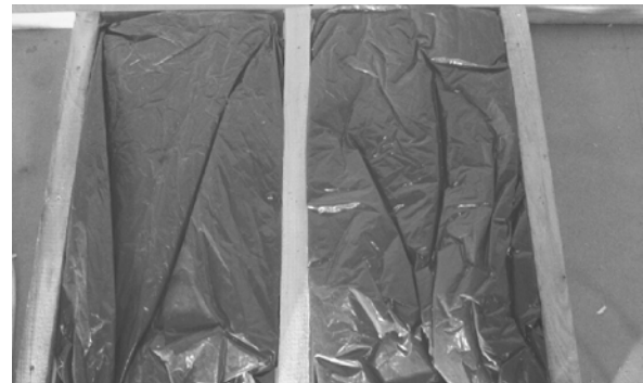
Fig. 3: Plastic foil bags at the rear of the cladding.
