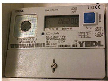
Figure 1: PV Generation Meter (showing total accumulated energy)
