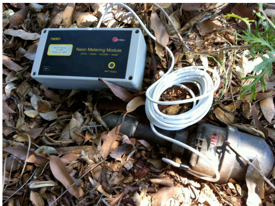
Figure 4: A Unidata logger and transmitter is connected to this V100 Elster water meter via a T-probe
