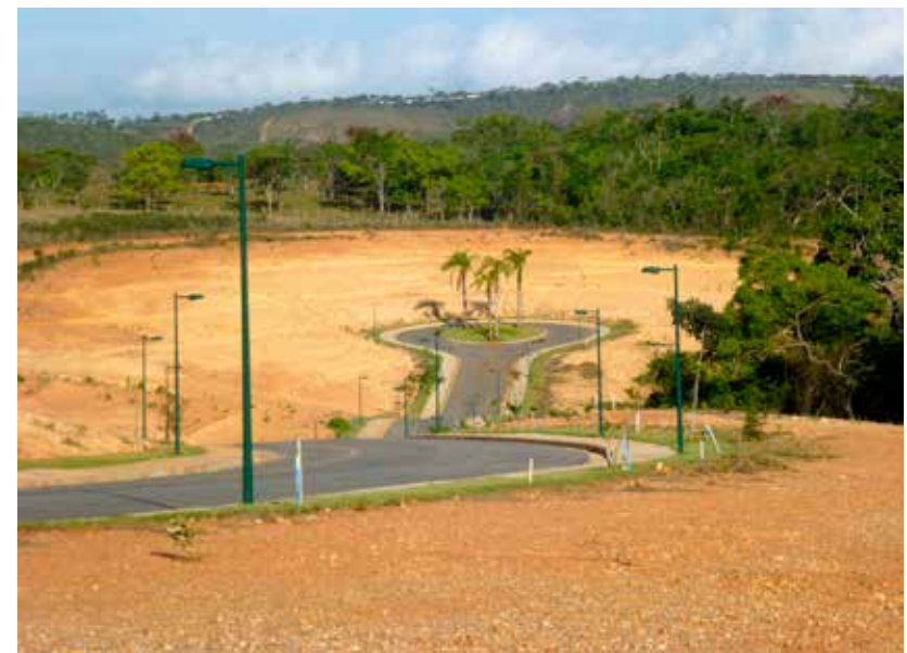
Land clearance for the construction of “Reserva Real,” north of Lagoa Santa
