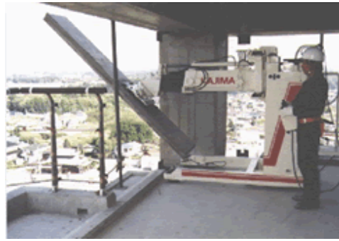
Figure 10. Example of a tele-operated robot, the so called Mighty Hand by Kajima Corporation.
