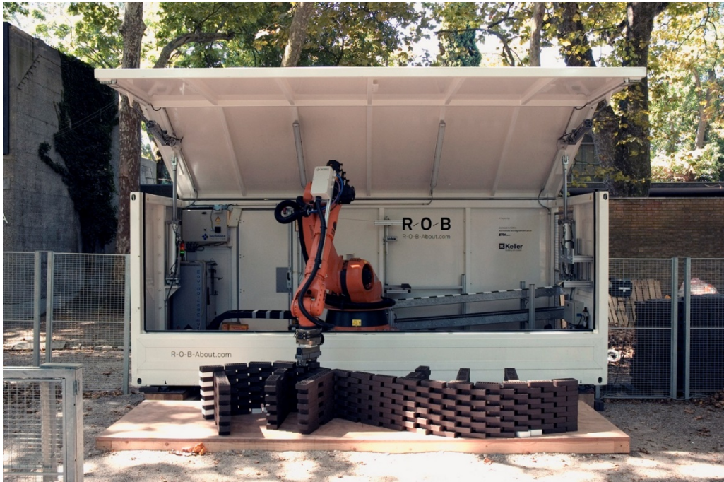
Figure 56. Experiment 3: ROB Unit assembling a segment of the Structural Oscillation installation (see Section 4.6.5).
